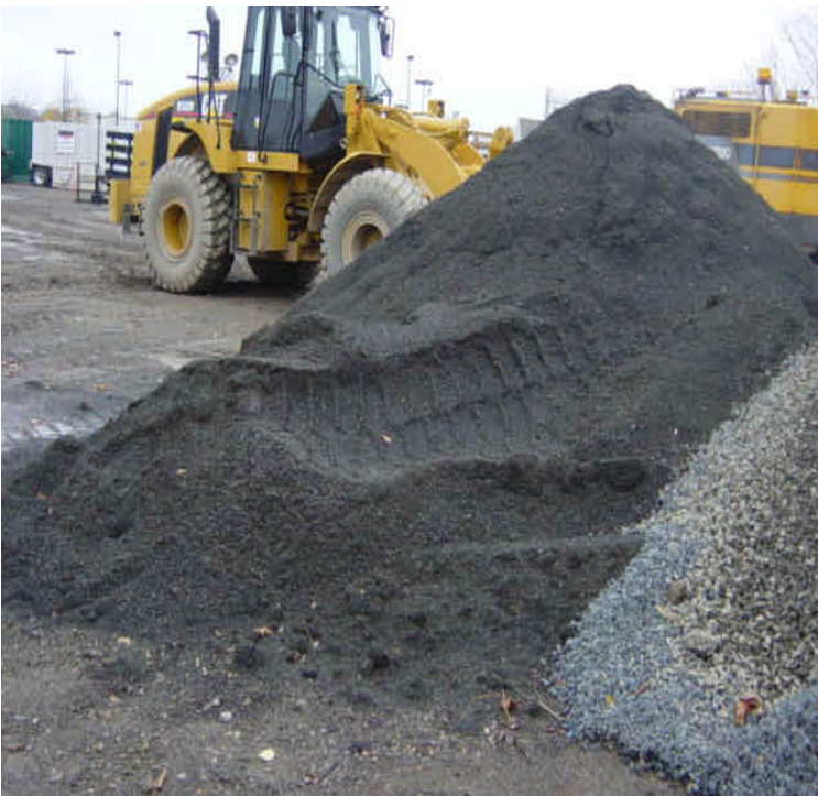
Material pile within the Kings Highway Laydown yard that is in close proximity to the adjacent resource area. Runoff from the pile contains a sheen and was collecting against the controls.
