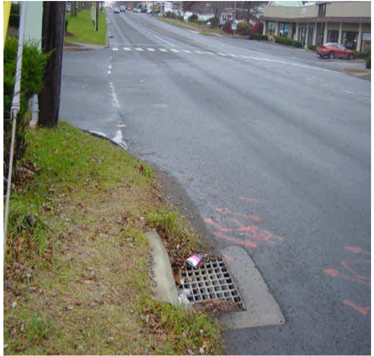
Photograph of an unprotected catch located downgradient of construction activities on Rt. 1 at the intersection with Buckley Ave.
