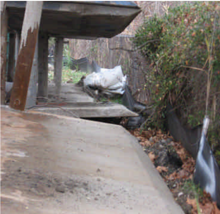
A portion of the perimeter controls on the side of the yard to adjacent to sensitive areas were overwhelmed by construction materials.
