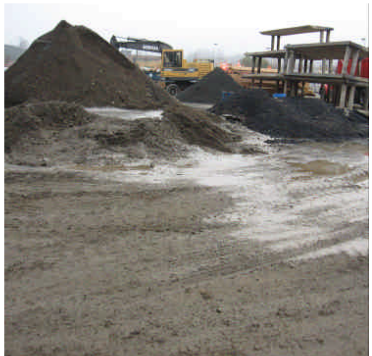
Photo of the concrete washout basin. The basin is not lined to isolate the washout from underlying soils, and it appears to be inadequately sized for storage.
