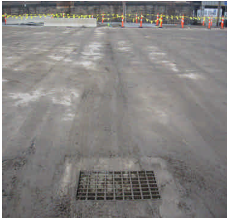
Photo of privately owned yard located immediately adjacent to trenching activities on Railroad Ave., south of Bostwick Ave. There is potential for sediment from construction activities to enter the catch basin.
