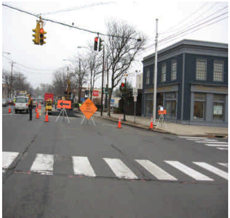
Construction activities on Rt. 1 at its intersection with Ruane St. The crews are applying asphalt to what appears to be the area excavated for the installation of Vault # 7533. This vault location is reflected in the 8/15/06 version of the D&M plans.
