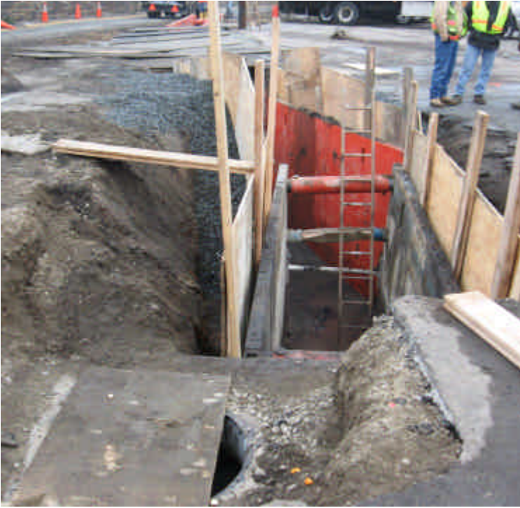
Photo of trenching activities at the intersection of Railroad Ave. and Howard Ave.
