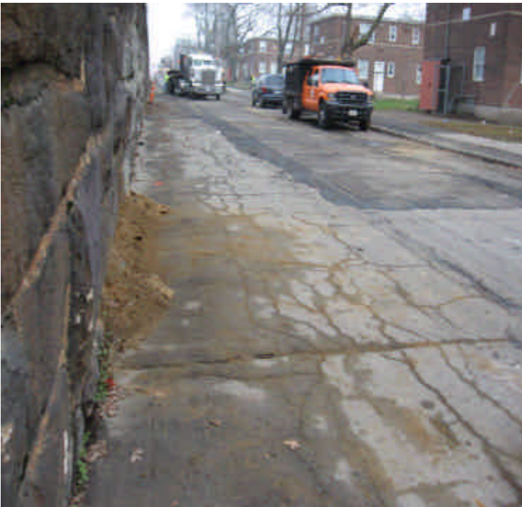
Photo of trenching activities on Railroad Ave. north of South St. Sediment in roadway should be removed as feasible.
