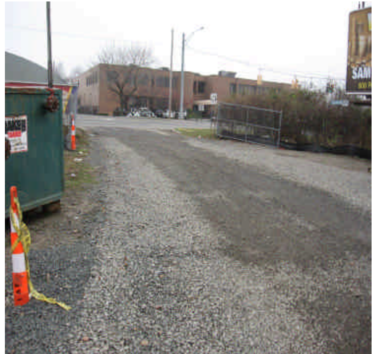
The construction entrance is well maintained and no evidence of sediment tracking was observed.
