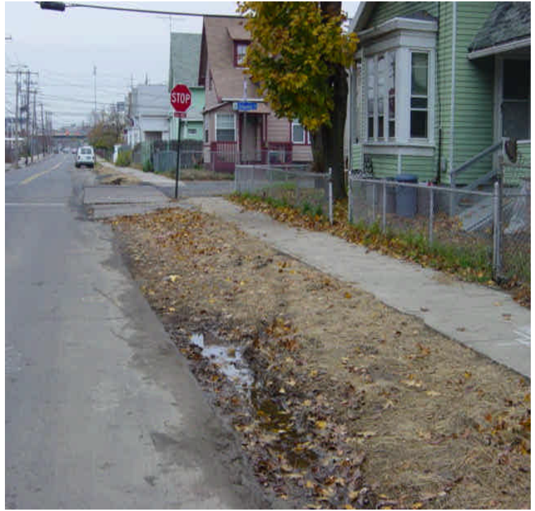
Photo of trenching location on Broad St. at its intersection with Atlantic Ave. that had adjacent tire ruts. Repair as needed.
