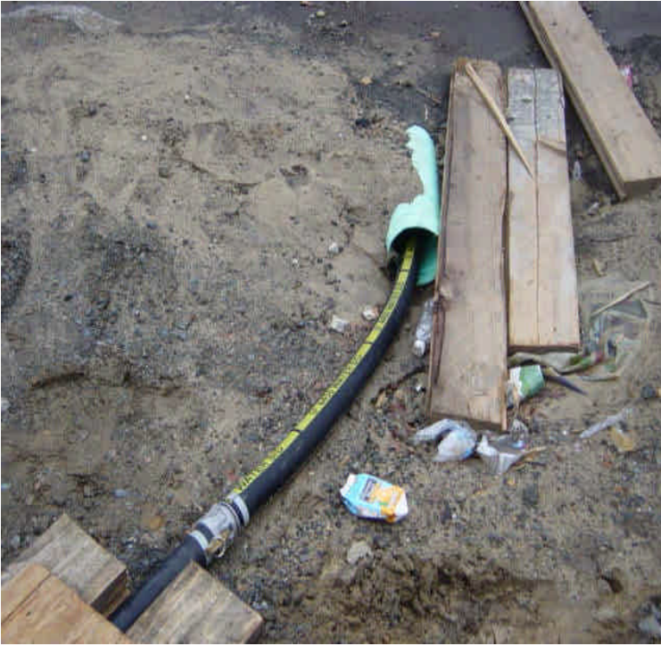
Filtered water from frac tanks is being discharged to sanitary sewer system via PVC pipe. The PVC pipe inlet does not have controls in place, potentially allowing sediment into the system.
