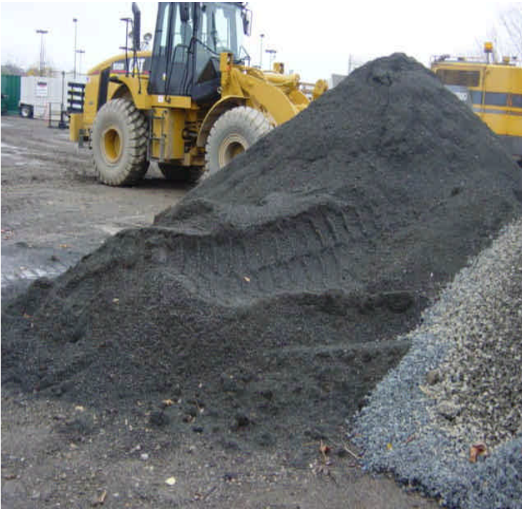
Material pile within the Kings Highway Laydown yard that is in close proximity to the adjacent resource area. Runoff from the pile contains a sheen and was collecting against the controls.
