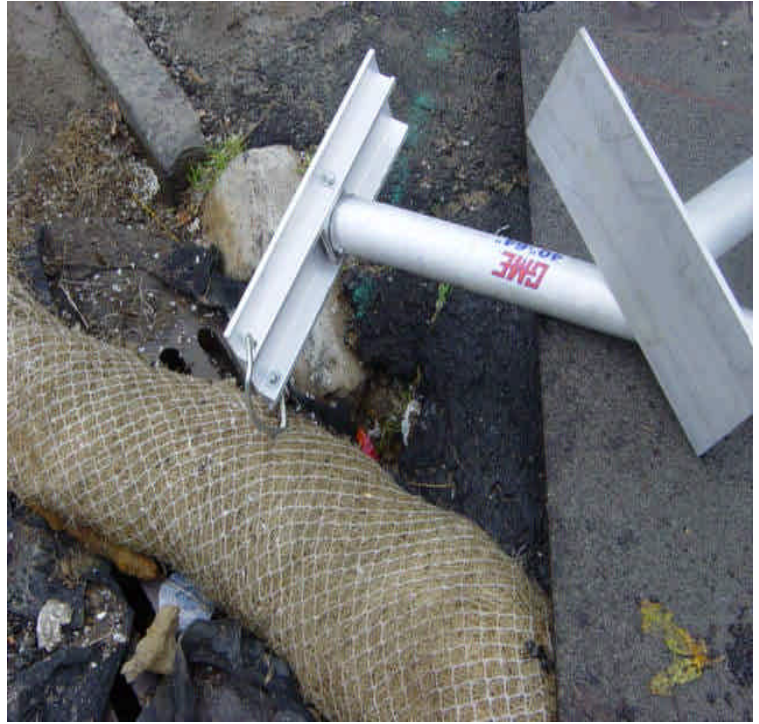
A catch basin located at the intersection of Railroad Ave. and Bostwick Ave. appears to be collapsing. Evaluate whether nearby trenching activities are responsible.
