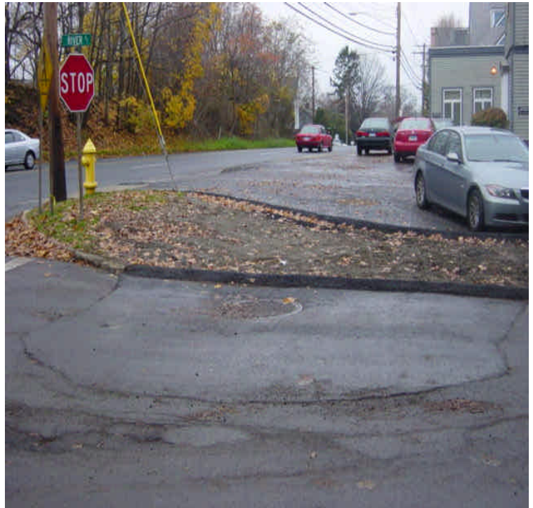
Location of Vault # 5430. Vault installation appears to be complete. Disturbed soils should be temporarily stabilized.
