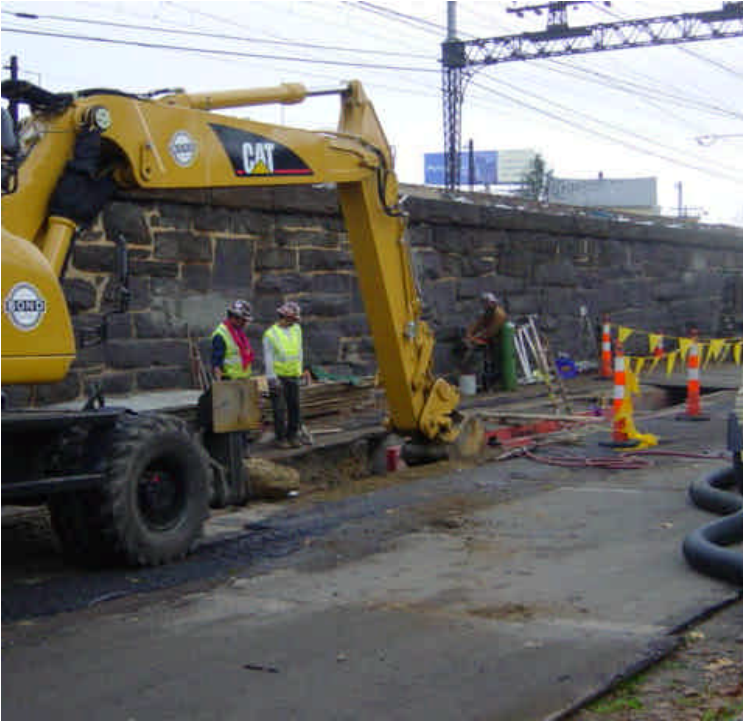
Trenching activities on Railroad Ave. near its intersection with Park Ave. Loose sediment was being swept from the roadway.
