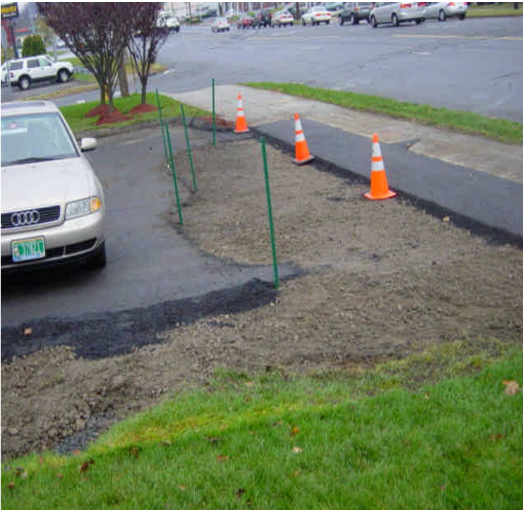
Location of Vault #7536. Vault installation appears to be complete. Disturbed soils should be temporarily stabilized.
