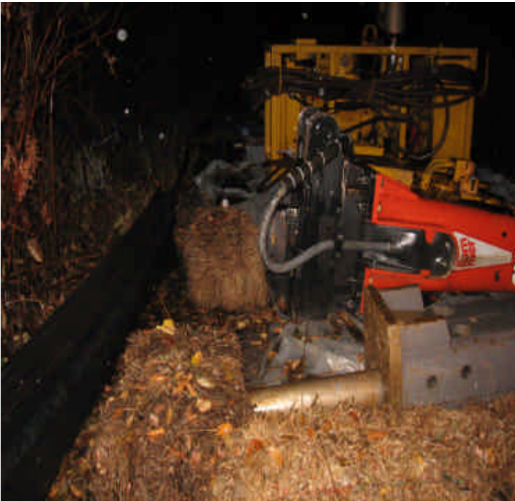
Photo of one of the attachment equipment storage area in the the King's Highway Laydown Yard. Please note that the containment area is not fully enclosed.
