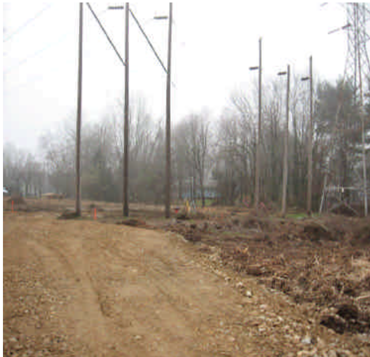
View of cleared ROW and constructed access road off Russell Ave. Some ruts were noted in the ROW due to soft soils.
