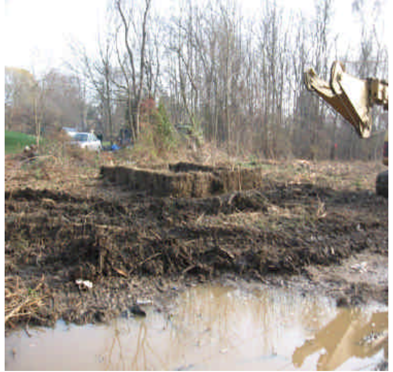
View of the dewatering area constructed near the first structure prior to drilling.
