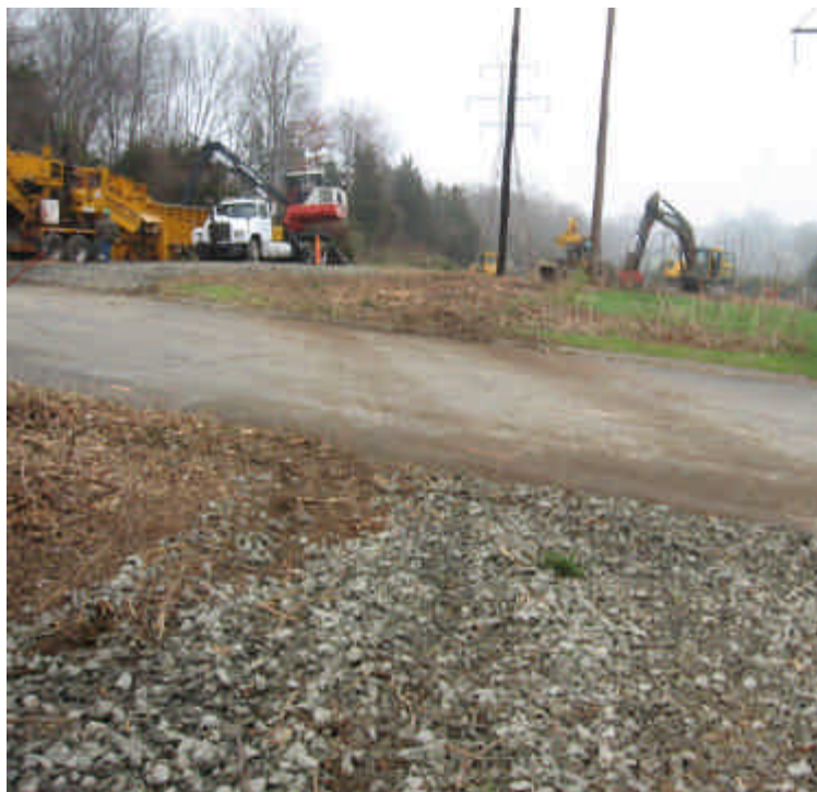
Stone access pads were installed at the access roads on both sides of Overland Drive. Some sediment tracking was noted during inspection. Silt saks have been installed within nearby catch basins.
