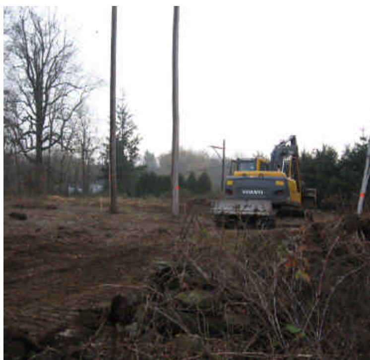
View of the clearing activities off Dogwood Road (east). The stone wall has been removed temporarily to provide access to structures.
