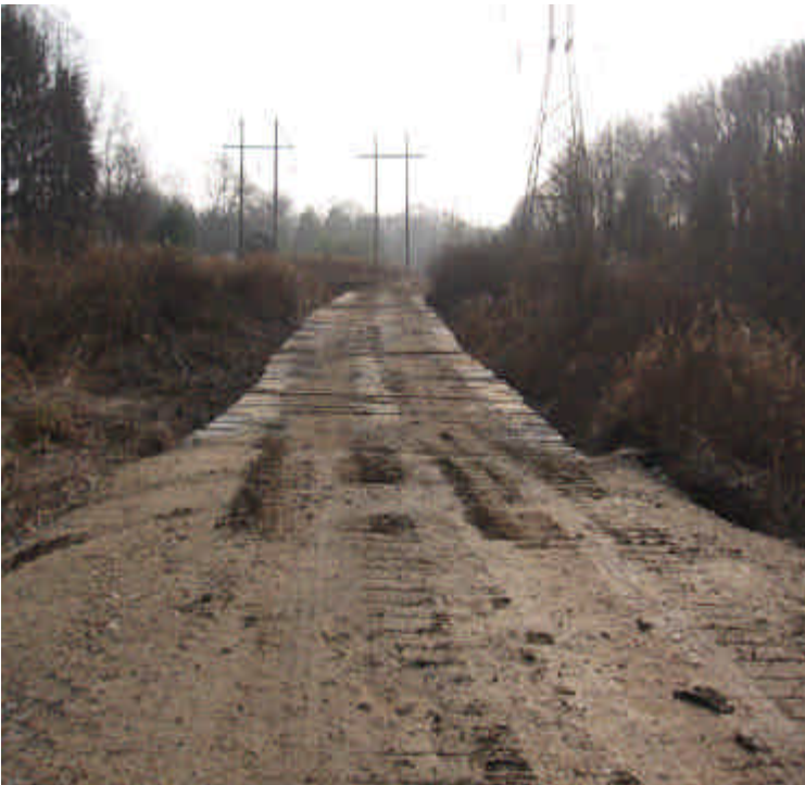
View of the wetland crossing constructed off Sunset Drive. This wetland is not federally jurisdictional.
