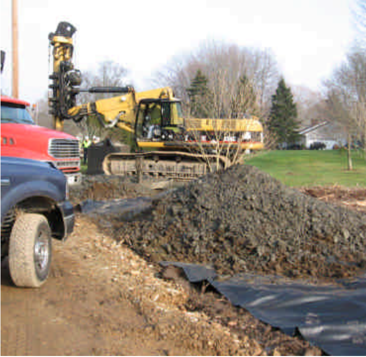
View of the foundation drilling off Sunset Drive. Spoil was placed on liner in an upland area. A silt sack was installed in the catch basin located immediately adjacent to the access road, and the fabric was pulled over the curb inlet to provide more adequate protection.
