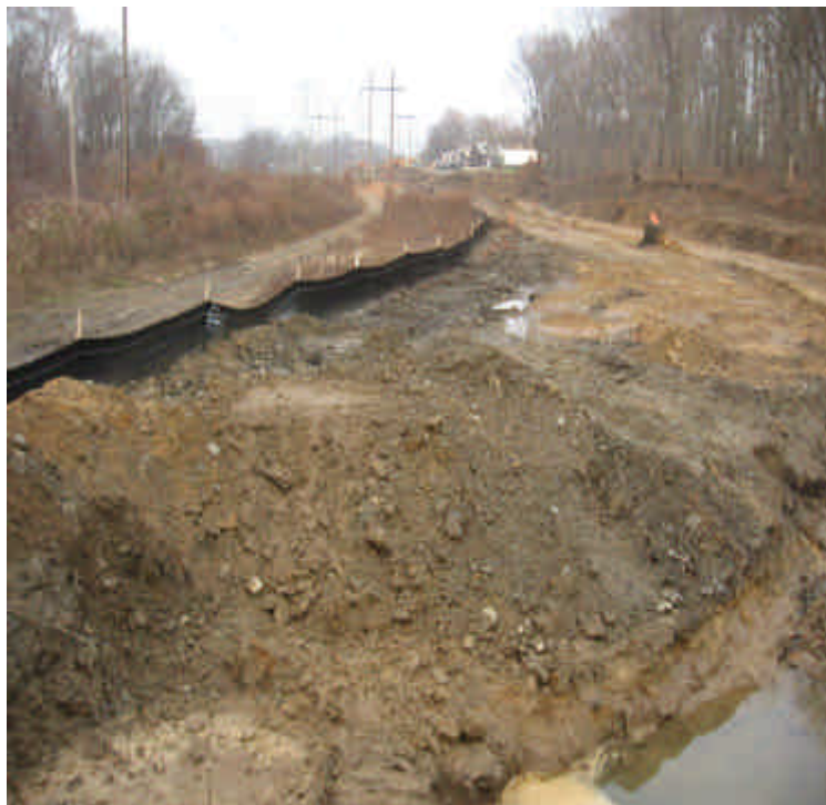
Activities associated with the relocation of Shelland Street continue. Silt fence has been placed along the work area.
