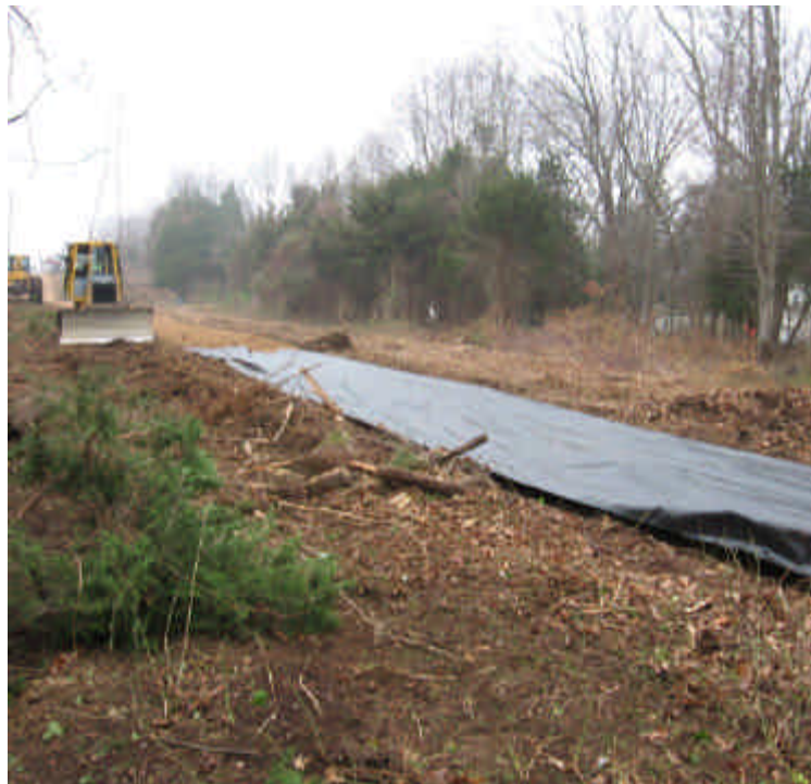
View of clearing activities and access road construction off Overland Drive (east).
