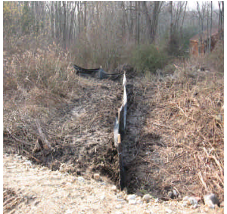
View of the silt fence installed along the wetland's edge within the ROW off Sunset Drive.
