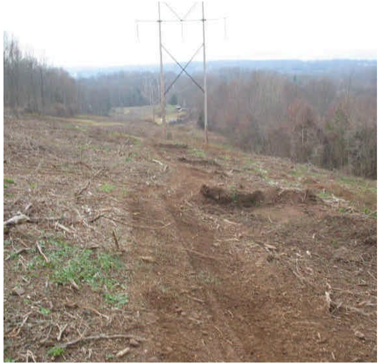
View of water bars in place along the slope in the ROW off High Hill Rd.
