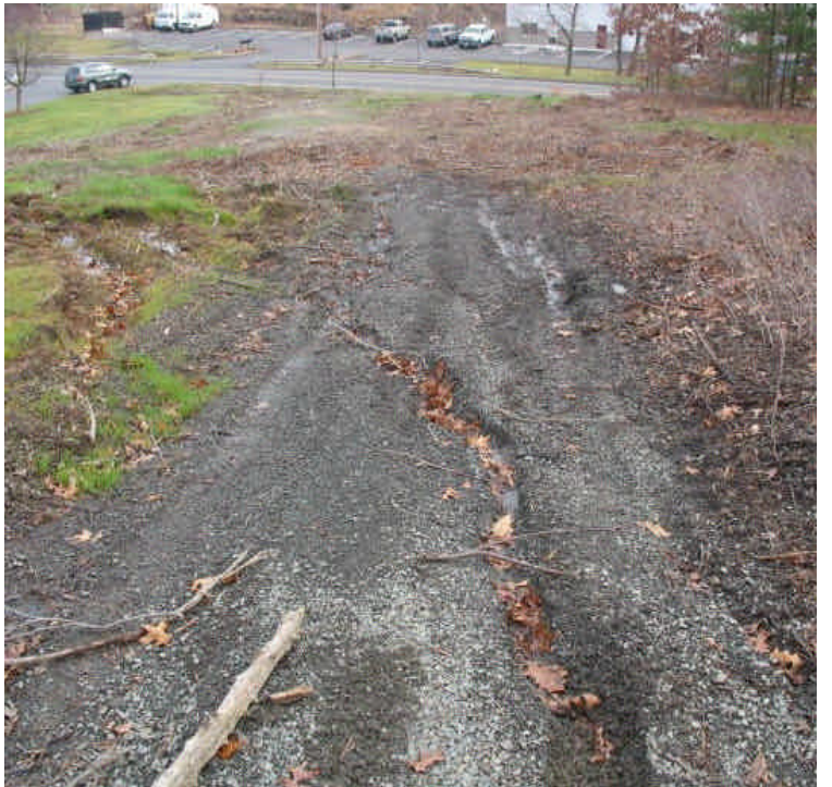
Erosive gully/washouts remain in the stone access road off South Turnpike.
