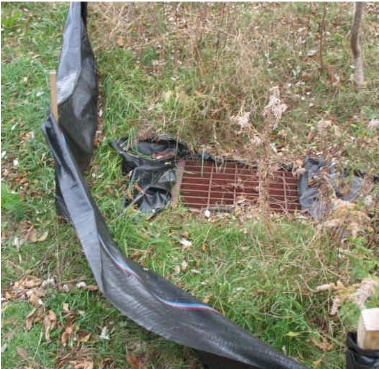
Catch basin controls in place off Stony Brook Rd.
