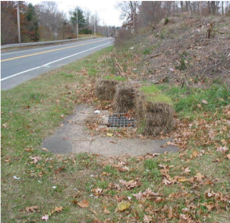
Catch basin protection off Rt. 68.
