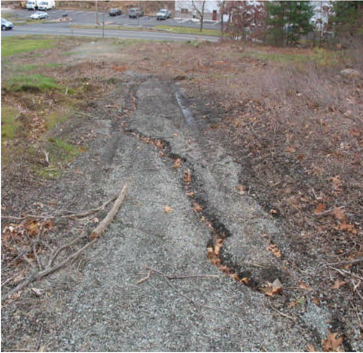
Washouts/erosive gullies noted in access road off of South Turnpike. Area will need some grading and stabilization/stormwater control.
