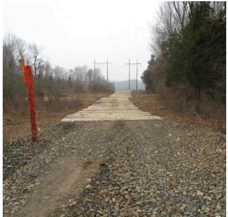
Non-jurisdictional wetland crossing area in the access ROW off Haddam Quarter Rd. Mats are in place and clean water was leaving the site.
