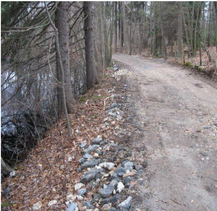
Erosion controls may need to be extended between the new access road and the pond off Haddam Quarter Rd. to prevent potential sedimentation.
