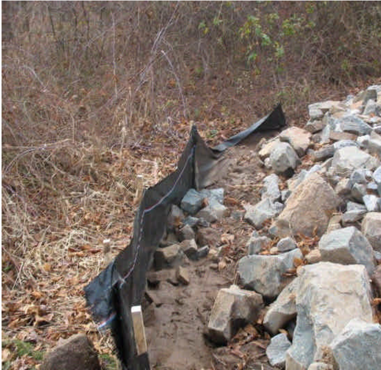
Riprap sediment trap and silt fence along the access road off Black Walnut Dr. Accumulated sediment should be removed and the silt fence maintained.
