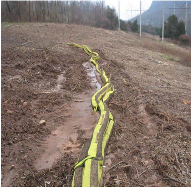
Bio-socks used to trap/filter slurry and sediment from dewatering efforts at Black Pond.
