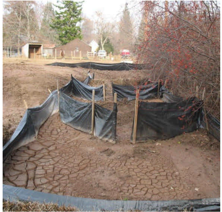
Slurry containment areas located in the ROW north of the contractor yard along Rte 17. Additional silt fence barriers were added to contain escaping sediment. Sediment is being removed and spread to dry.
