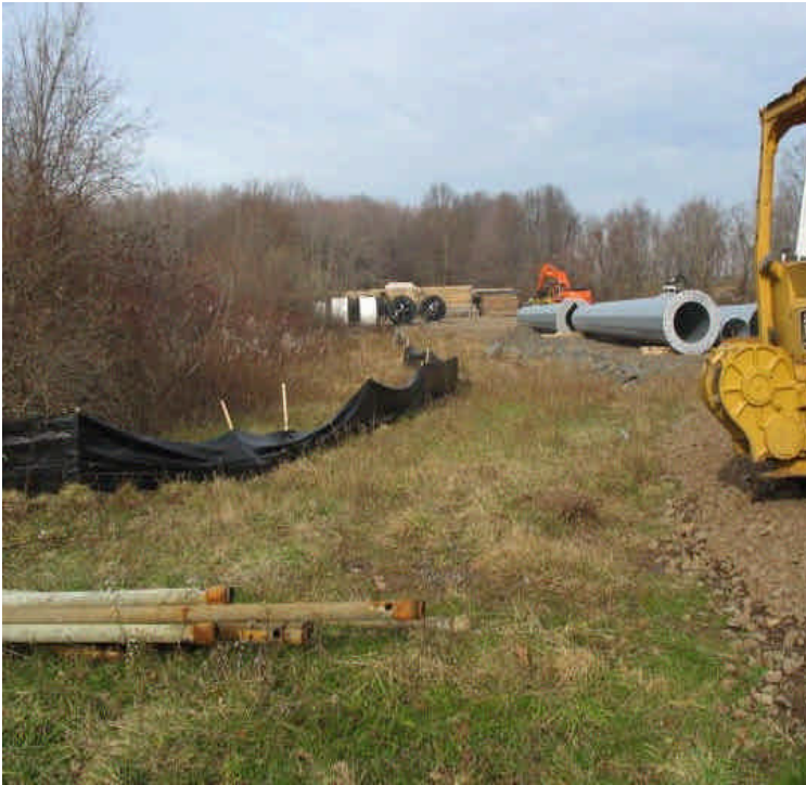
Silt fence should be re-stapled along the pond in the contractors receiving yard. Equipment should be parked/stored as far from wetlands as feasible (100ft if possible).
