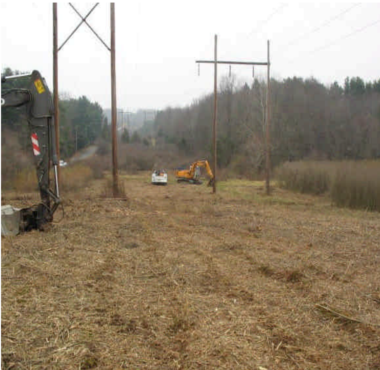
View of clearing activities off Little Lane. Continue to retain vegetation whenever feasible based on the D&M plan.
