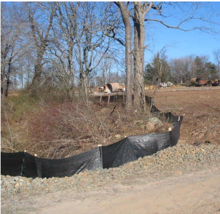
Silt fence remains in place along the drainage ditch at the contractor receiving yard & staging area.
