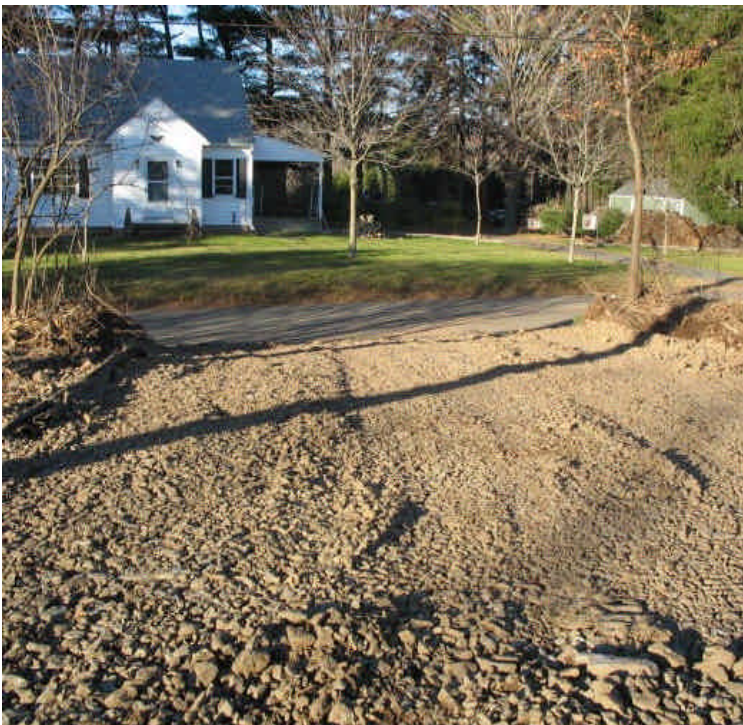
Entrance off Little Lane. No sediment tracking was noted. Continue to monitor stone pad and roadway.
