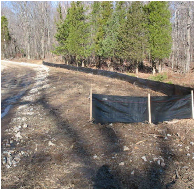
Silt fence was extended off Haddam Quarter Rd, at the end of the access road and ROW. Extended silt fence will provide additional stormwater filtration.
