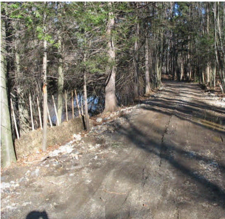
Erosion controls may need to be extended between the new access road and the pond off Haddam Quarter Rd. to prevent sedimentation.
