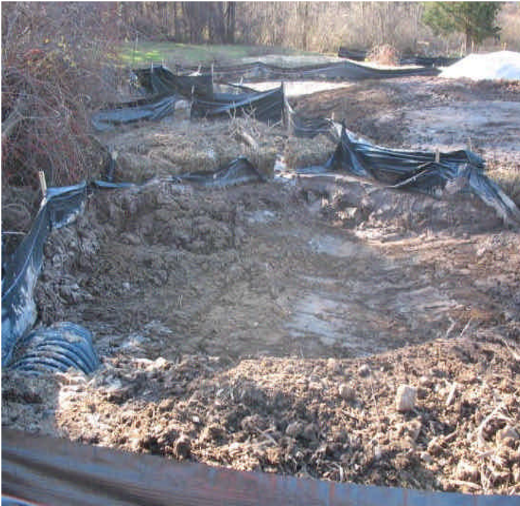
Slurry containment areas located in the ROW north of the contractor yard along Rt 17. Additional silt fence barriers were installed to contain sediment. Sediment is being removed and spread to dry. Ensure that future run-off over the dried, exposed soil is controlled.
