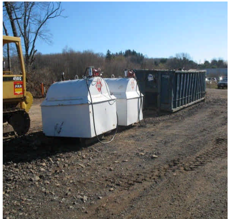
Fuel tanks stored at the contractor yard. Relocate dumpster within the yard to an area greater than 100-feet from the wetland if feasible.
