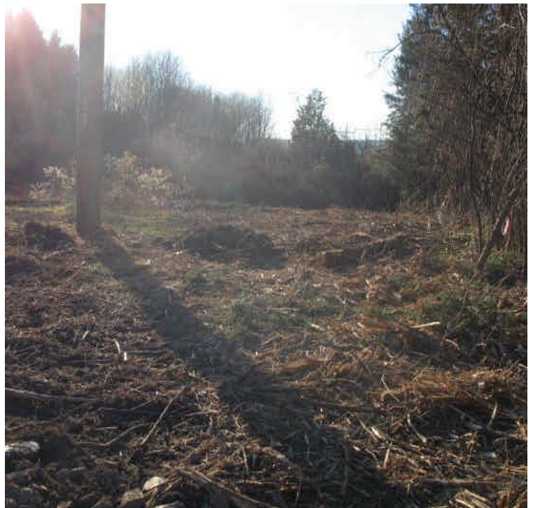
View of clearing activities off Little Lane. Continue to retain vegetation whenever feasible based on the D&M plan.
