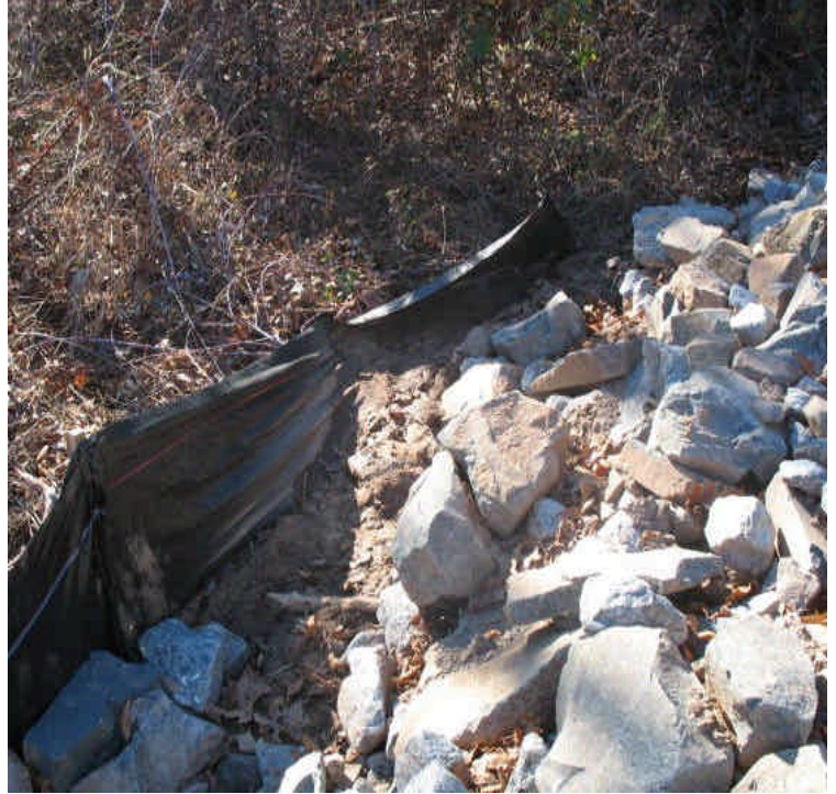
Riprap sediment trap and silt fence along the access road off Black Walnut Dr. Accumulated sediment should be removed and the silt fence maintained.
