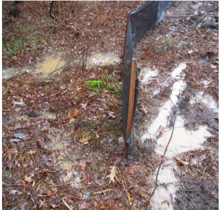
Turbid run-off was noted flowing around the silt fence and off site at Haddam Quarter Rd, at the end of the access road and ROW. Extend silt fence and provide additional filtration.
