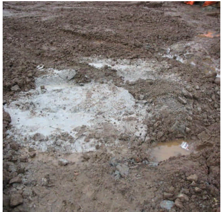
A small concrete washout was noted outside the designated washout area along Rte. 17. The concrete should be removed and disposed of
