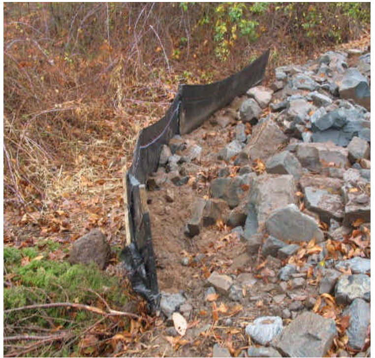
Riprap sediment trap and silt fence along the access road off Black Walnut Dr. Sediment was cleaned out but should be placed upland, away from the silt fence.
