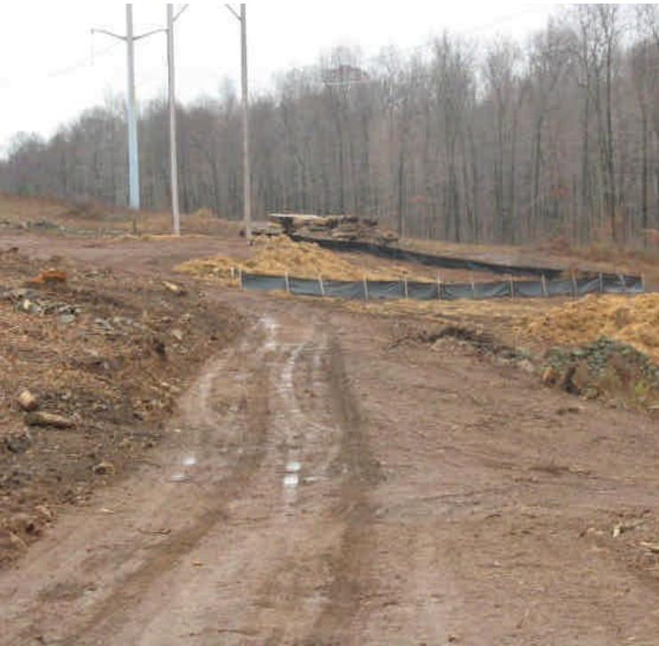
Cleared area north of Beseck SS. New silt fence added at drill sites in preparation for the work.
