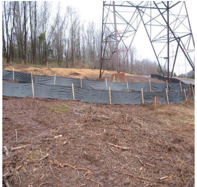
Silt fence/haybale barrier along the access road adjacent to Black Pond in preparation for drilling in the area.
