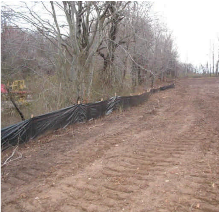
Silt fence remains in place along the drainage ditch at the contractor receiving yard & staging area.
