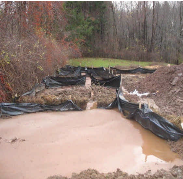
Slurry containment areas located in the ROW north of the contractor yard along Rte 17. Additional silt fence barriers were added to contain escaping sediment.
