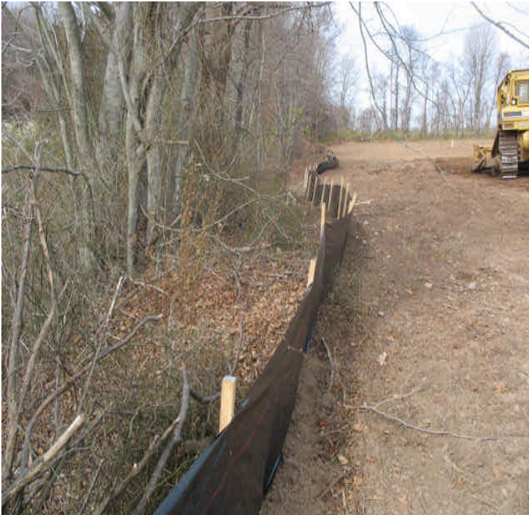
Silt fence was installed along the drainage ditch at the contractor receiving yard & staging area.
