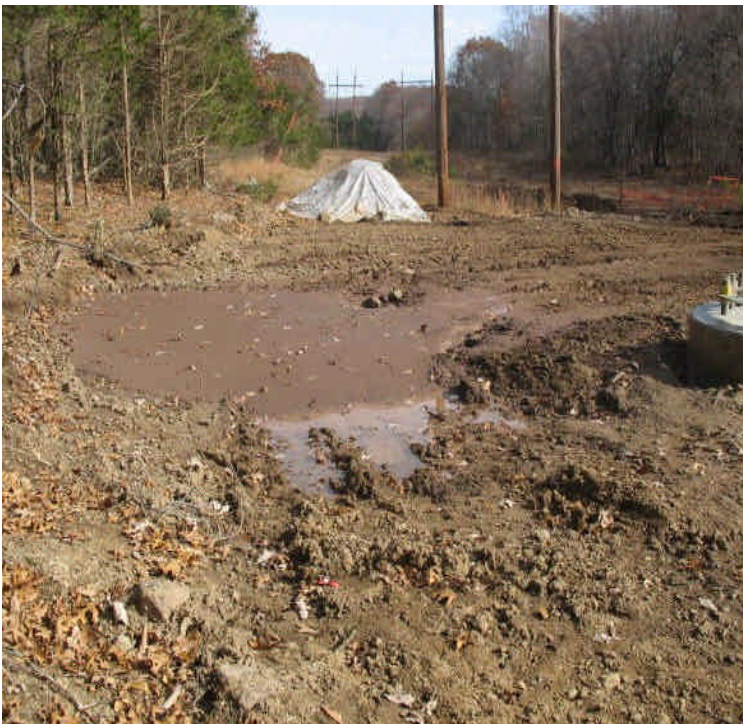
Slurry storage and drying area from foundation drilling/dewatering off Black Walnut Dr.
