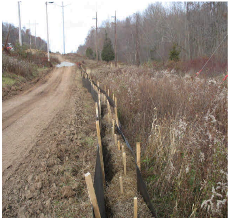
Silt fence/haybale barrier along the access road adjacent to the wetland near Beseck SS.
