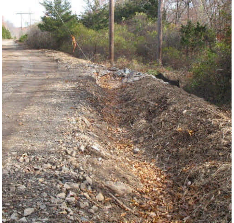
View of the recently installed swale and riprap sediment trap along the access road off Black Walnut Dr.
