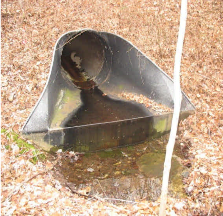
Water was noted flowing through the culvert under the access drive due to the recent rains. Sediment issues were not observed.
