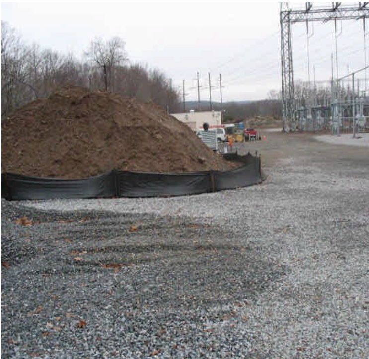
The remaining soil stockpile is surrounded by silt fence. Run-off remains contained by the crushed stone on site.
