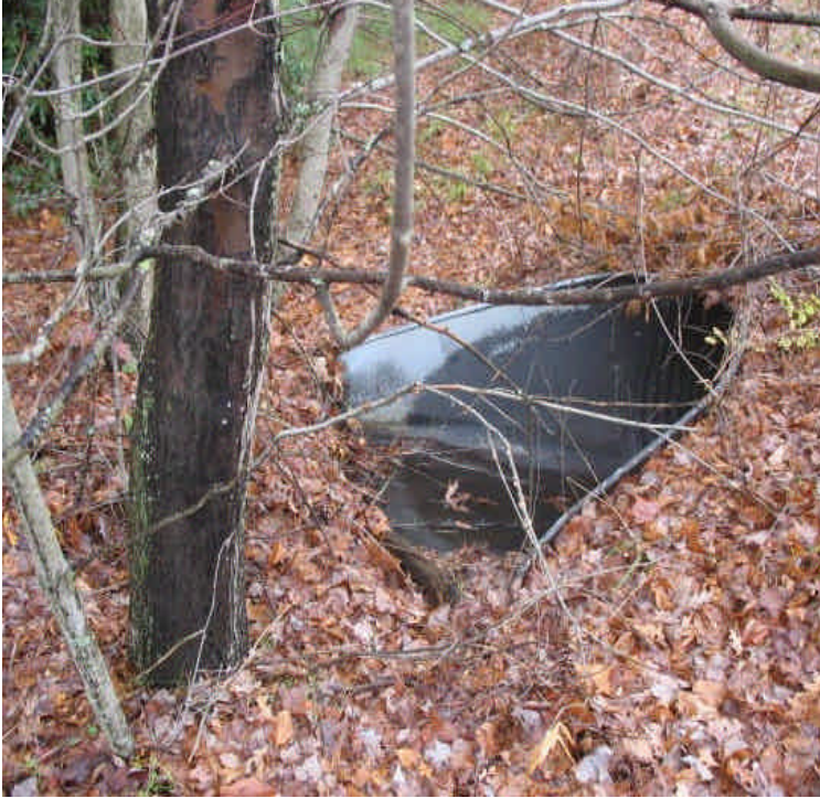
Water flow was noted through the culvert under the access drive due to the recent rains. Sediment issues were not observed.
