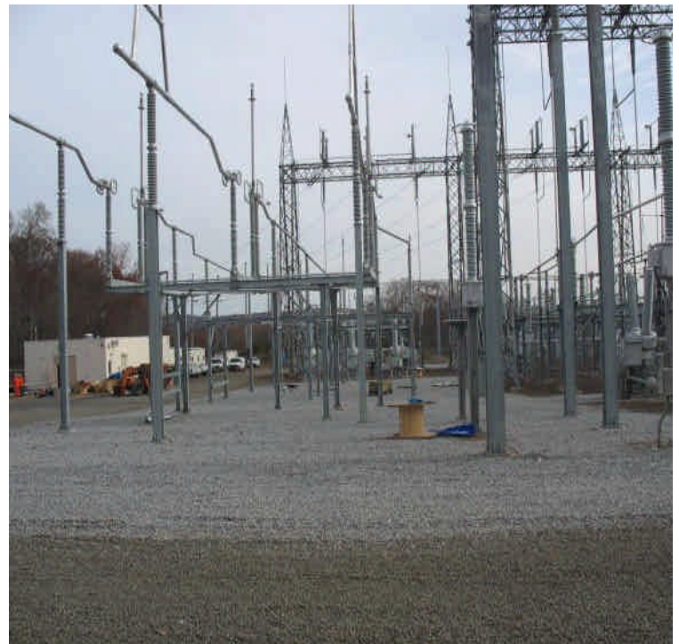
Foundation installation is complete; the site has been graded and stabilized with stone. Work continues on structures.
