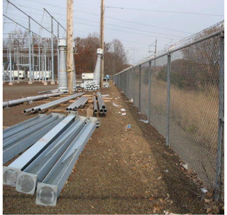
Silt fence was removed from the perimeter and site is stable. Most soil disturbing work on site is complete at this time.
