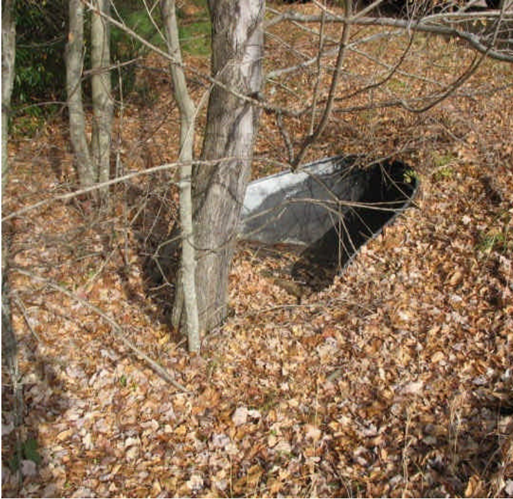
No water was flowing under the access drive, no sediment noted from the rain last week.
