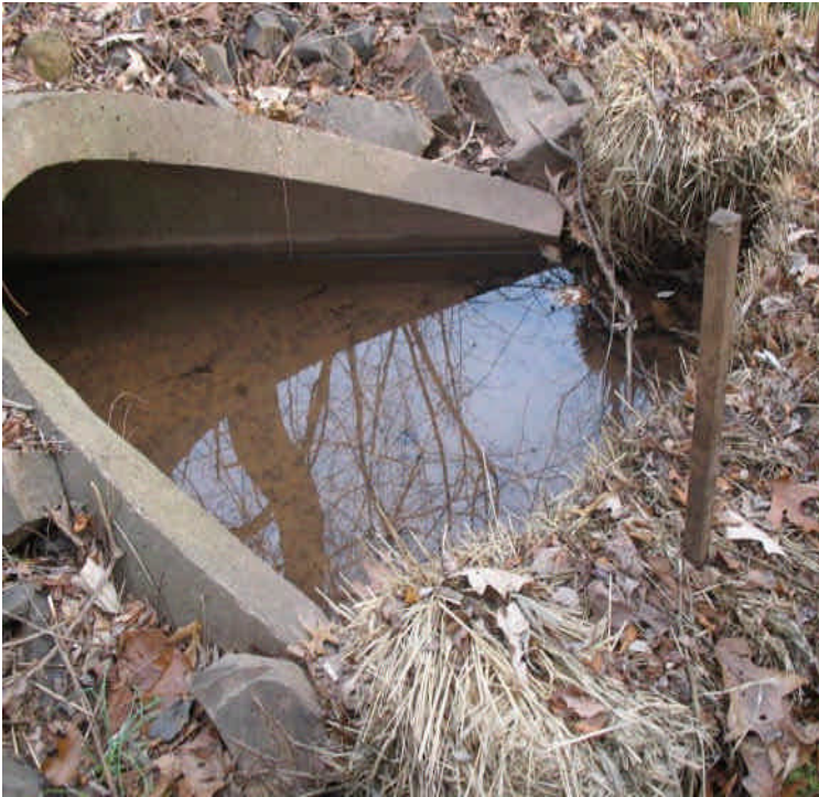
Storm drain outlet across Carpenter Lane contained settled sediment with clear water standing water at the pipe.
