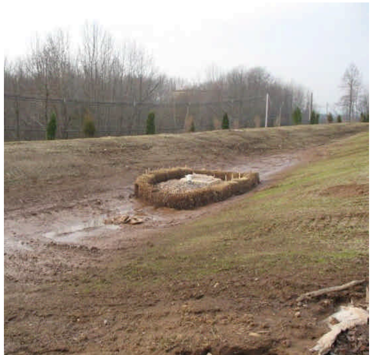
Some grass growth was noted on the seeded slopes of the detention basins due to the warm weather. Additional/alternative controls are still recommended to protect the inlet as turbid water may pool over and into the system.
