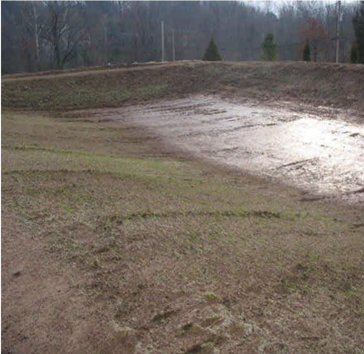
Grass growth noted on detention basin slopes due to the warmer weather. Continue to monitor for stabilization.
