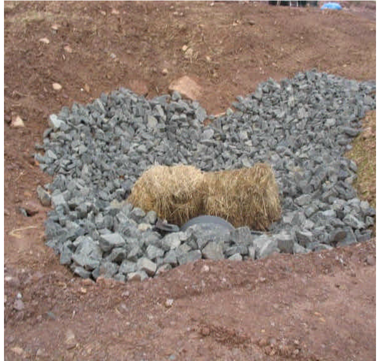
View of the culvert under the new access road. Haybales are still in place and sedimentation was not noted. Beseck and 1A contractors are sharing the joint access road.
