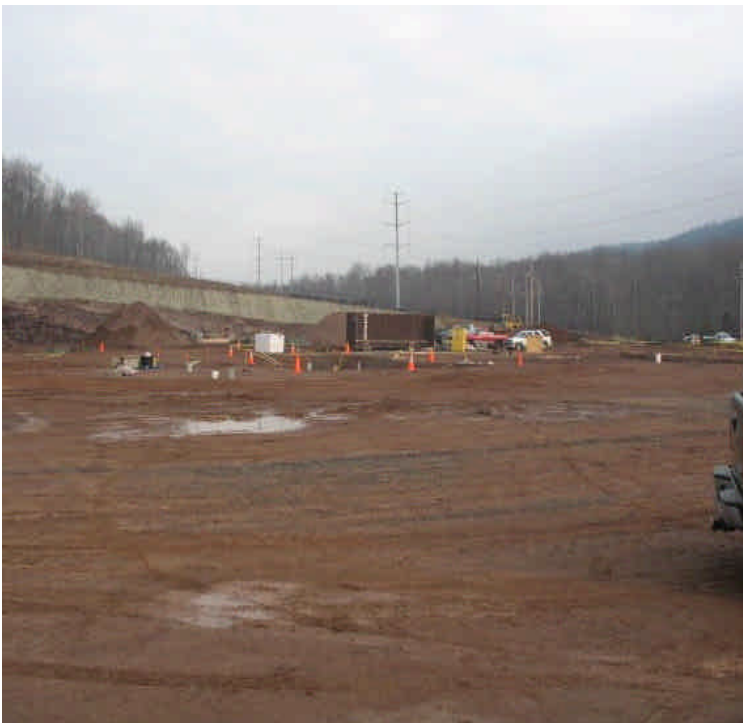
View of entire site looking from south to north. Work on foundations continues.
