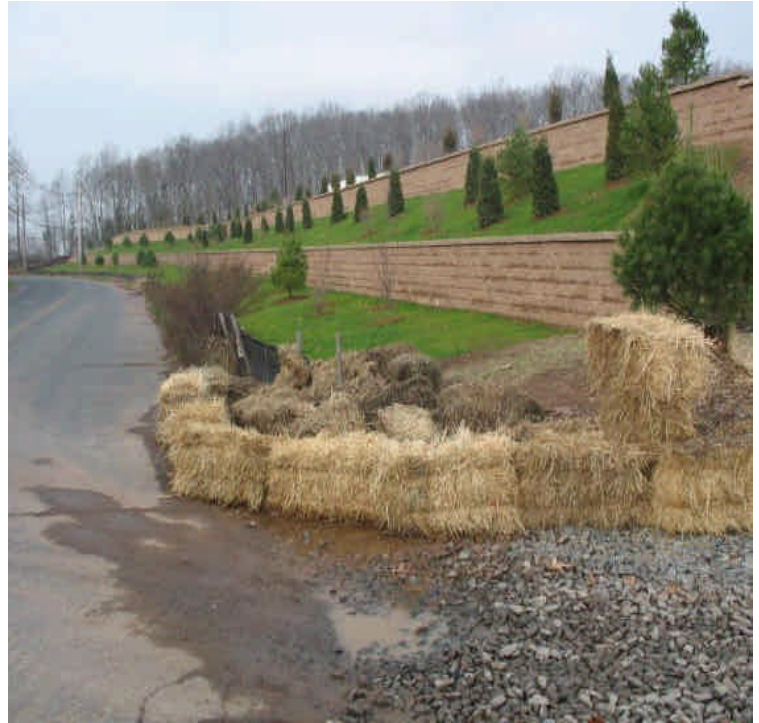
View of Carpenter Lane and retaining walls. Even with recently installed, additional controls, minor amounts of turbid-runoff were still noted leaving the site
