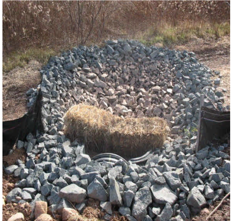
A riprap sediment trap is now in place at the culvert outlet. The old ROW access road is now closed off and contractors share the Beseck entrance. Haybales were installed to control sediment.
