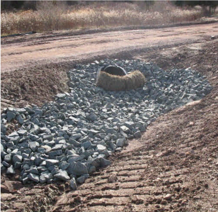
Culvert inlet at the ROW access road from Beseck. Riprap & haybales were in place to reduce sedimentation.
