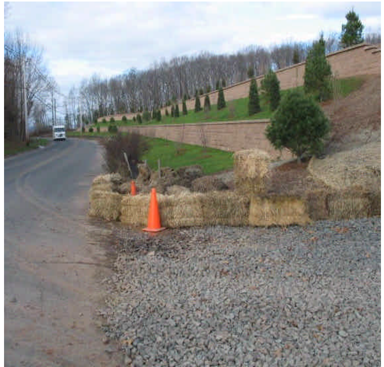
View of Carpenter Lane and retaining walls. New haybales were installed, the stone entrance was regraded, and the roadway was swept. Minor sediment tracking was noted.
