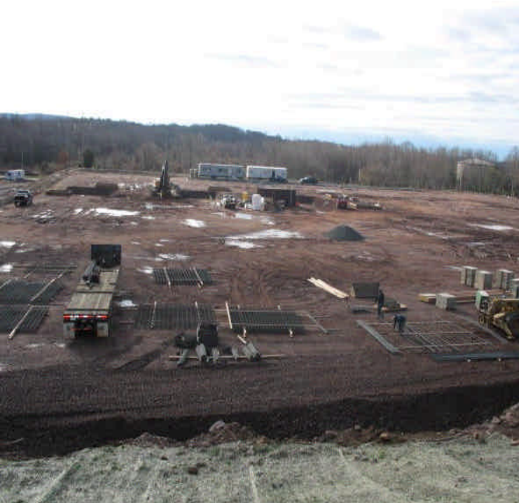
View of entire site looking from north to south. Foundation excavations are underway.
