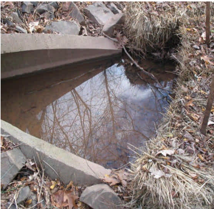
Storm drain outlet across Carpenter Lane had settled sediment on the bottom with clear water leaving the pipe.
