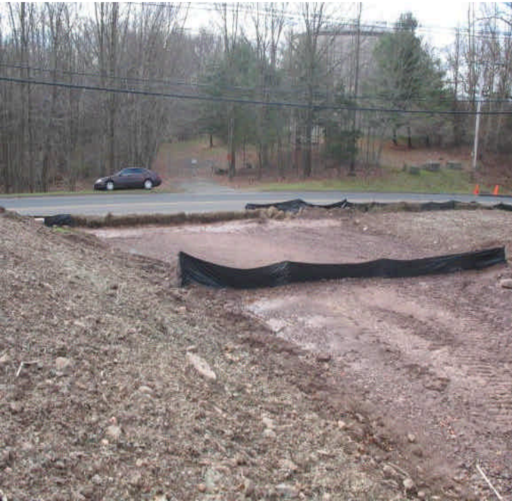
New entrance off Carpenter Lane. Additional haybales and silt fence were installed.
