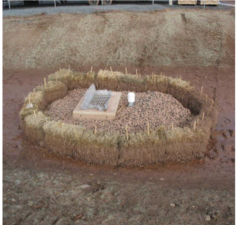
Efforts were made to control the new detention basin inlet until grass cover can establish. However, it appears water is pooling over the controls during large rain events, allowing turbidity to enter the system. Additional/alternative controls are recommended.
