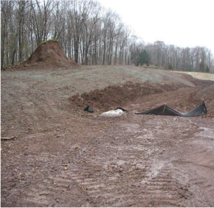
Old Zolnik entrance at Carpenter Lane. New haybales were added and the area was graded and hydroseeded.
