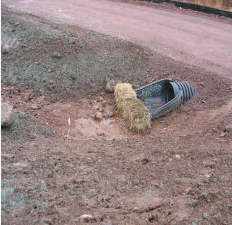
New culvert inlet at the ROW access road from Beseck. Haybales were in place to reduce sedimentation.
