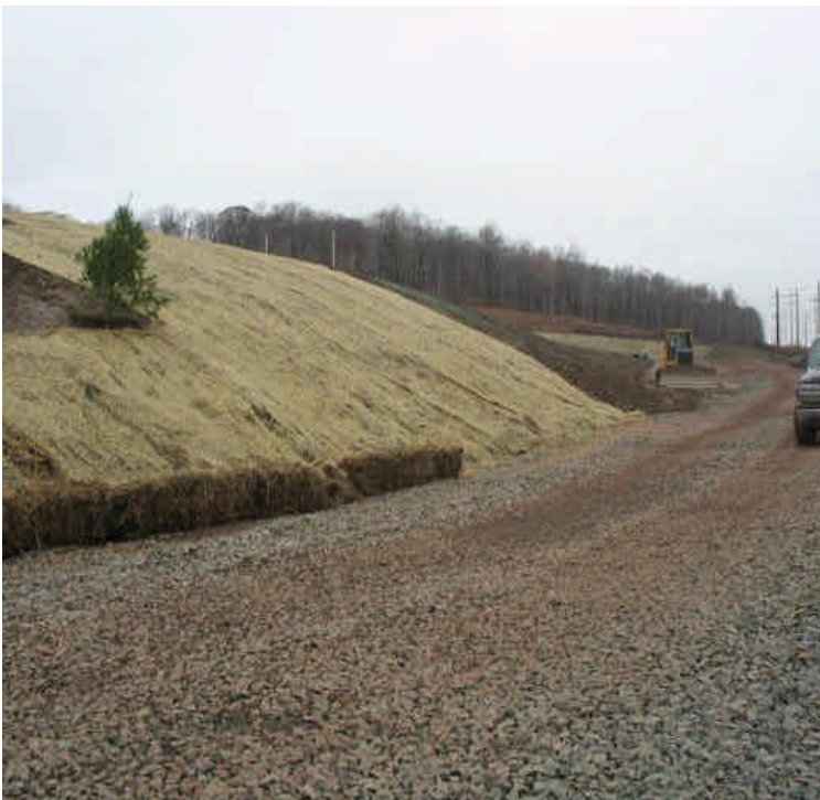
Erosion control mats were installed along steep slopes. Remaining exposed soil surfaces were hydroseeded.
