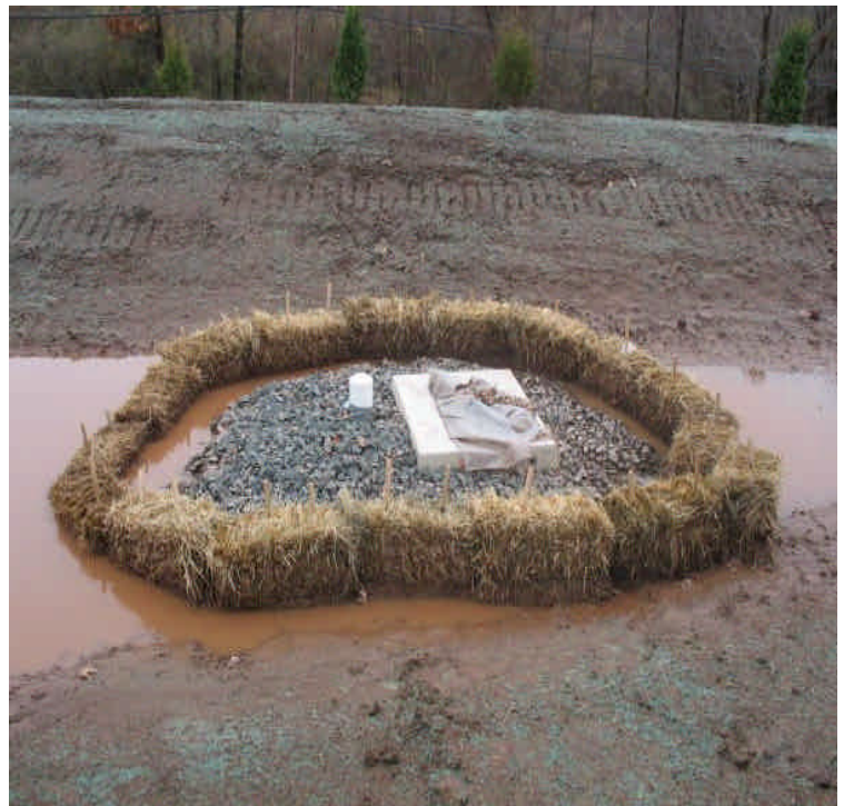
Efforts were made to control the new detention basin inlet until grass cover can establish. However, vegetative cover is not expected prior to the winter and additional controls are recommended to remove turbidity.
