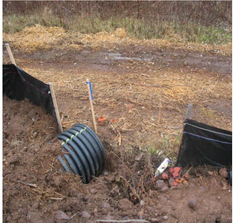
Culvert outlet installed under the new access road. The road connect the Beseck entrance to the ROW and will be used jointly. A sediment trap will still be needed at the outlet.
