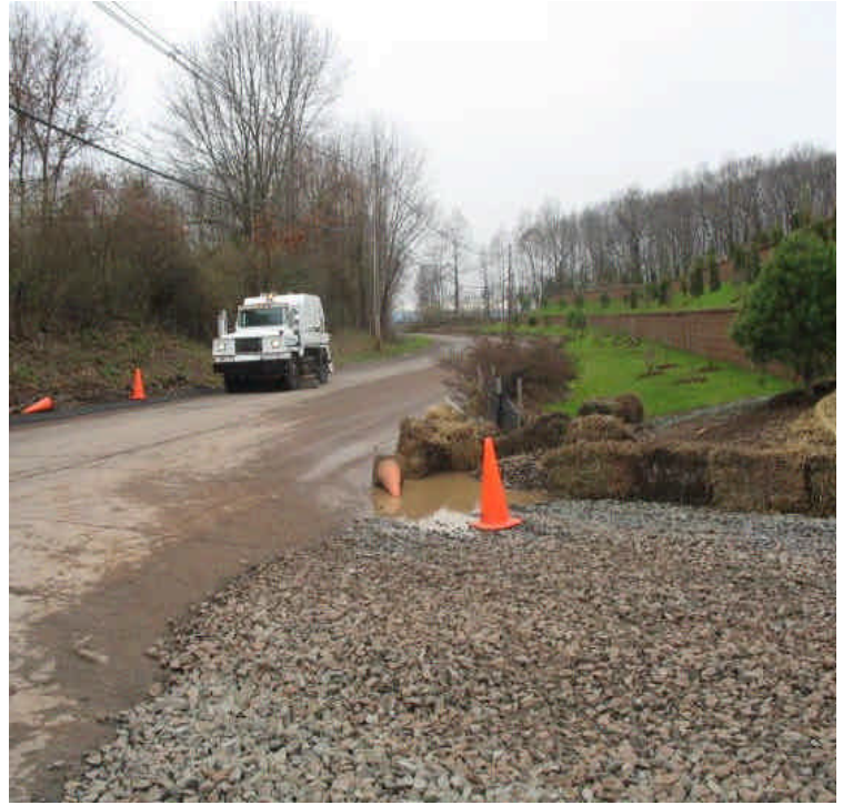
View of Carpenter Lane. Street sweeping was occurring and the stone entrance was reggraded but turbid run-off was still reaching the roadway.
