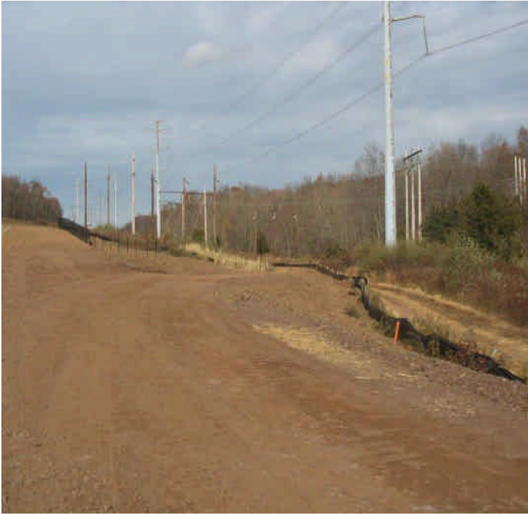
New ROW access from Beseck at finished grade; new silt fence installed.
