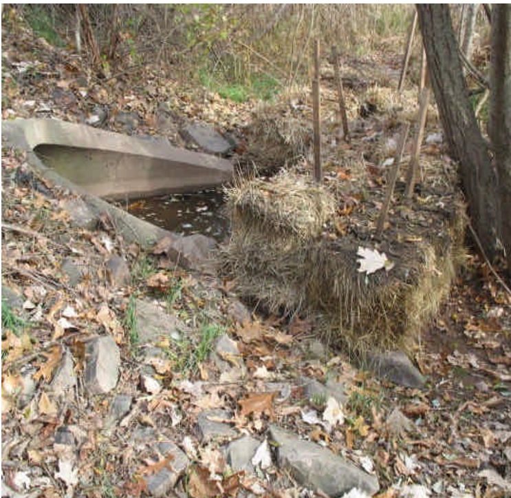
Sediment has settled out in the bottom of the storm drain outlet. A good haybale barrier is in place.
