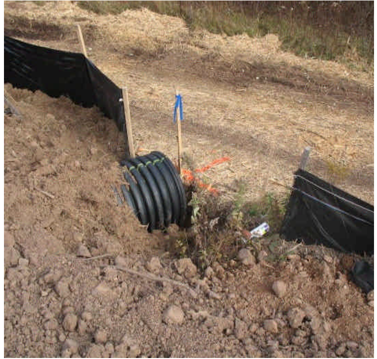
A culvert was installed under the new access road. The road connects the Beseck entrance to the ROW and will be used jointly. A sediment trap will still be needed at the outlet.
