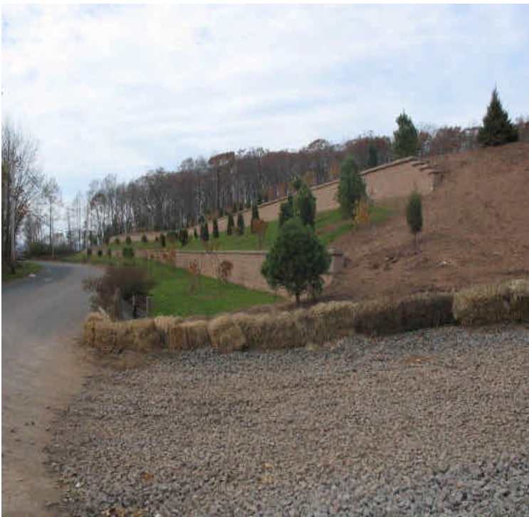
Stone site entrance at Carpenter Lane. Stone is fairly clean of sediment. Final landscaping was complete along the new retaining walls.
