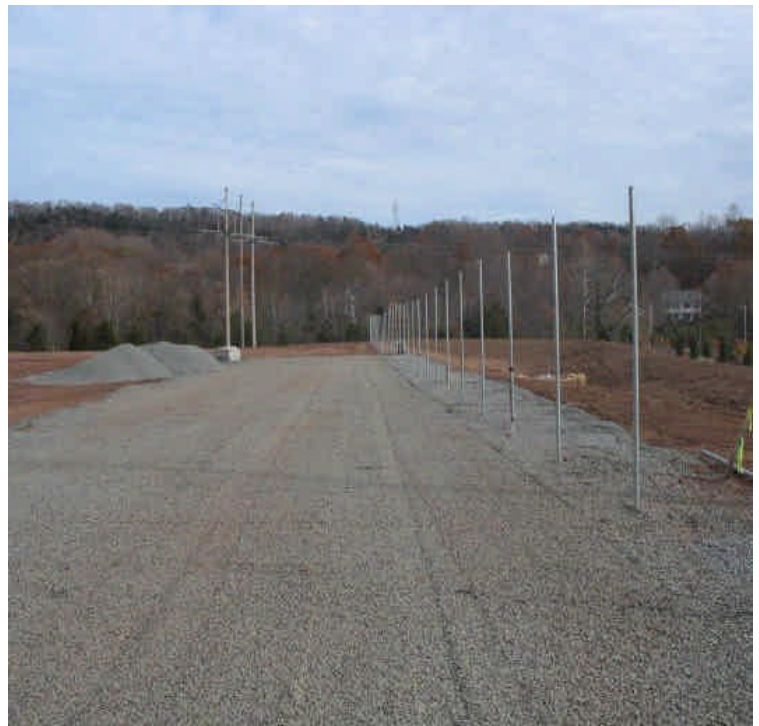
Crushed stone was added to finished areas above the new retention basins. This will also help to reduce exposed surfaces on site.
