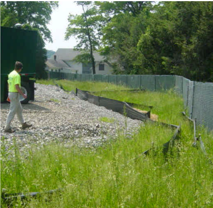
A portion of the controls within the Sherwood Ave. lay-down yard have been overwhelmed. The controls should be re-established
