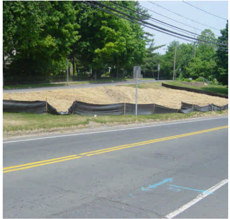
Photo of the vault #5 area. The surface has been top-dressed with a hard pack material and hay mulch. A small portion of the silt fence is slumping and should be re-established.
