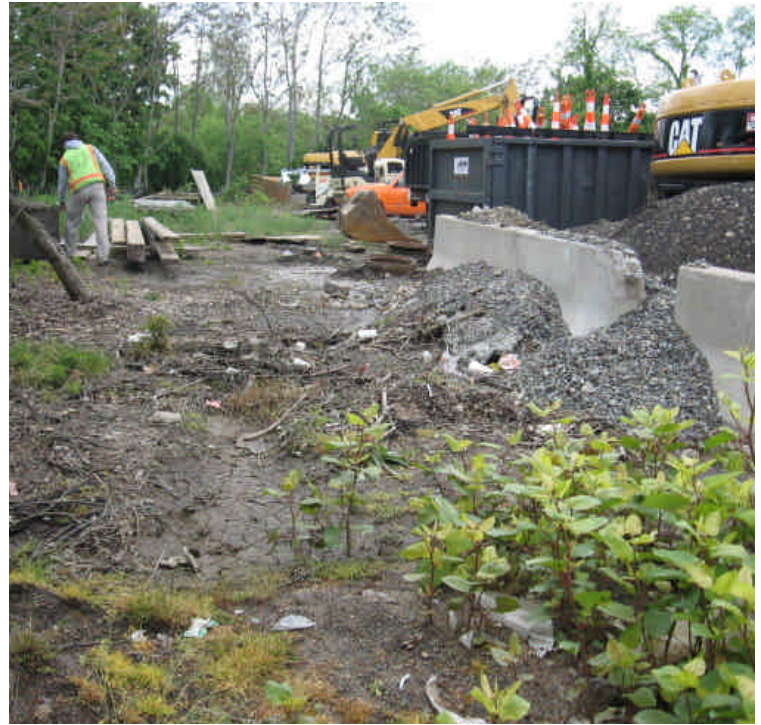
Photo of storage materials that have overflowed their containment bins, and of the drainage path of migrating sediment within the Imperial Ave. lay-down yard. Sediment and materials still remain within the perimeter of the yard.
