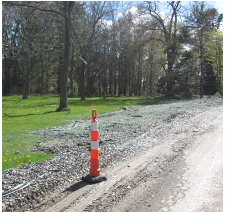
The majority of stone was removed, regraded, and hydroseeded (and mulched) along the edge of the access road to the Sherwood Island lay-down yard.
