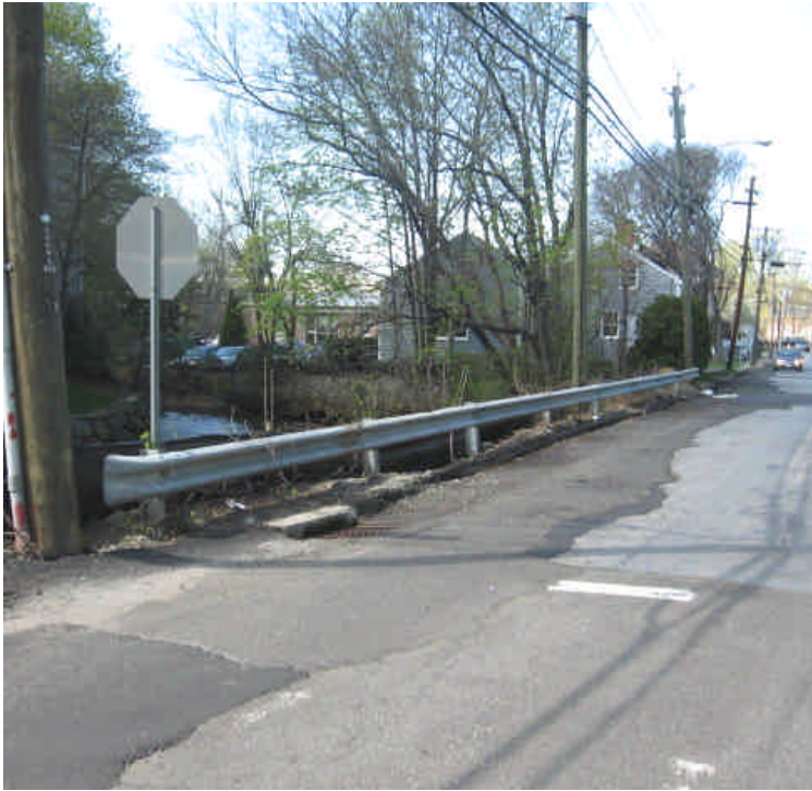
Photo of Imperial Ave. near sta. #260. The area is no longer active but erosion controls remain between the roadway and the creek for future work.
