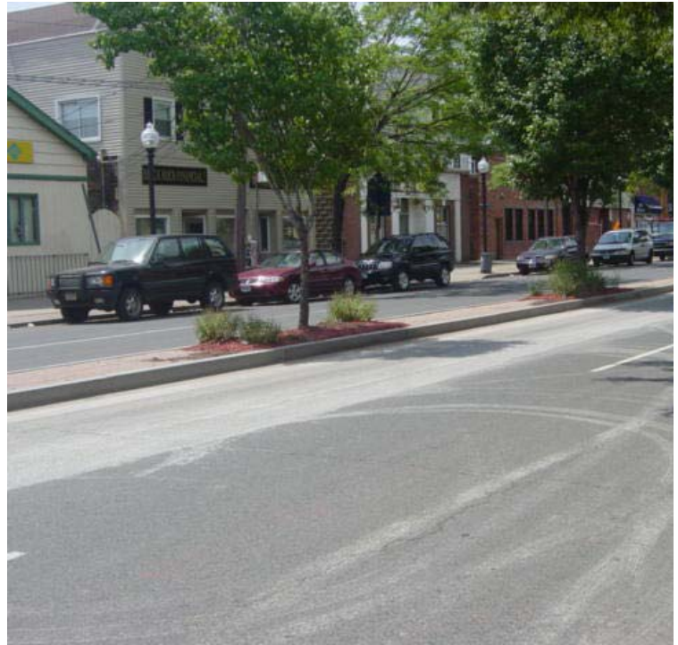
Saw cutting was recently performed near sta. #672 to #674 and some of the dried slurry/dust remains along the roadway. Prevent slurry from entering catch basins and sensitive areas by quickly attending to it as it is generated. Sweep as needed.
