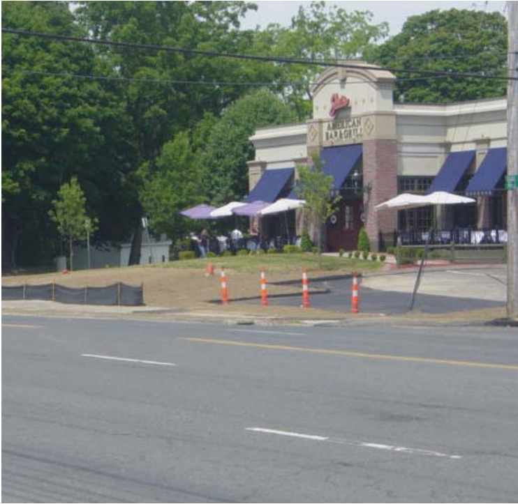
Vault #36 has been backfilled and requires seed and mulch for final restoration. Silt fence remains along the downgradient side of most of the work area.
