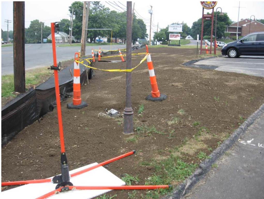
Soils remain exposed at vault # 37 location. Seed and mulch should be applied as soon as feasible to prevent erosion/gullyng and potential sediment migration during storm events. Erosion controls remain in place.
