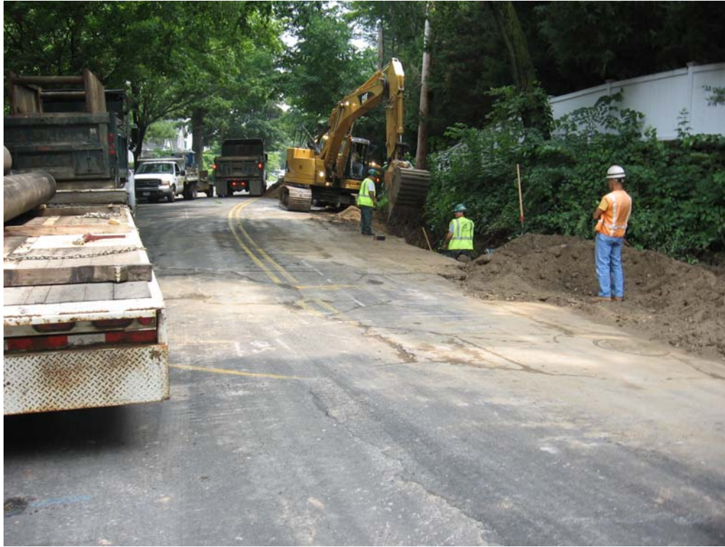
Photo of utility relocation activities along Pequot Ave. All catch basins were adequately protected. Sweep roadway as necessary.
