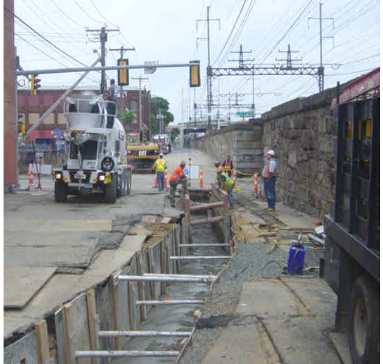
View of open trench and backfilling activities along Railroad Avenue near sta. #789.
