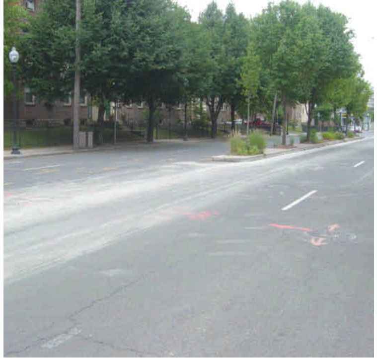
Saw cutting had recently occurred near sta. #675 to #680 and some of the dried slurry/dust remains along the roadway. Prevent slurry from entering catch basins and sensitive areas by quickly attending to it as it is generated. Sweep as needed.
