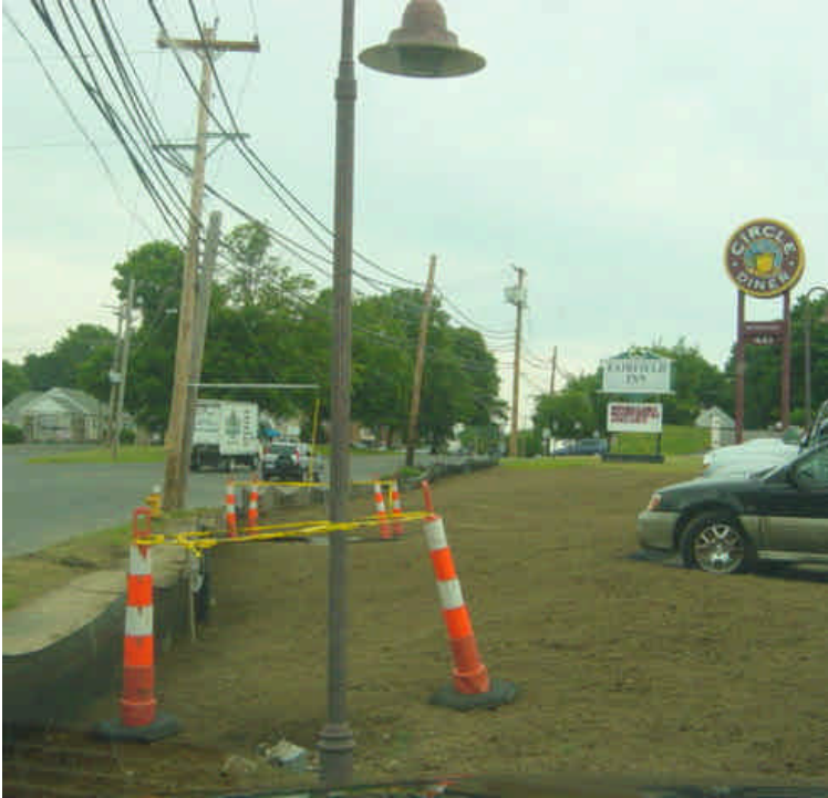
The area of exposed soil near vault #37 has been graded and topsoil was applied. The area needs to be seeded and mulched. Silt fence remains in place.
