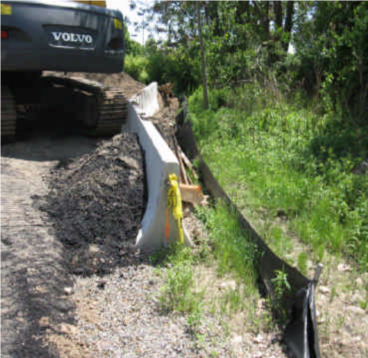
The majority of the compromised silt fence within the King's Highway lay-down yard has been re-established. The portion of the fence in the foreground of the photo required additional reinforcement when feasible.
