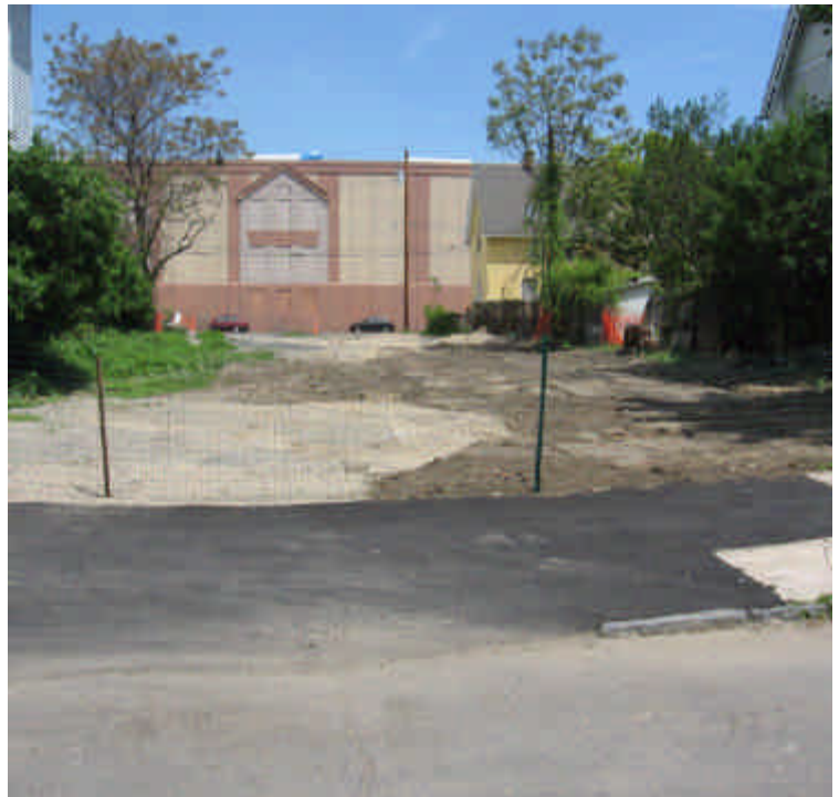
Topsoil is being added to the former trenching location between Broad and Main St. in an effort to restore the area.
