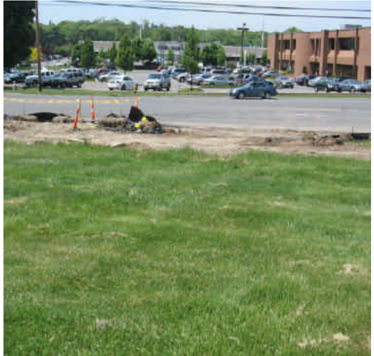
Activities continue at the vault #37 location. Access to the construction area has been obtained through an entrance in the erosion controls. Recommend re-establishing controls or placing haybales at the close of each day to prevent sediment migration during heavy rain events.
