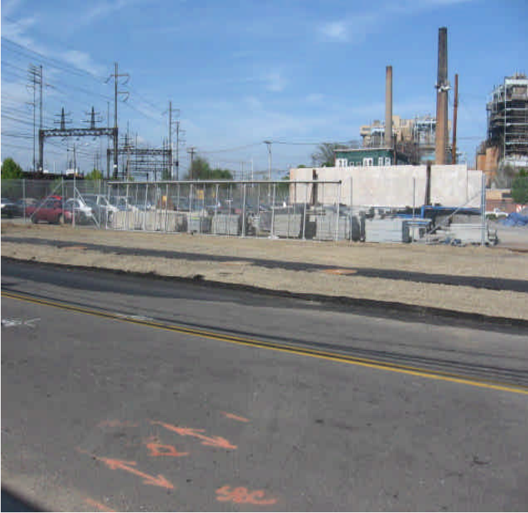
Photo of the vault #49 location. A hard pack material has been applied as a surface layer. Final stabilization/restoration measures should be implemented when feasible.
