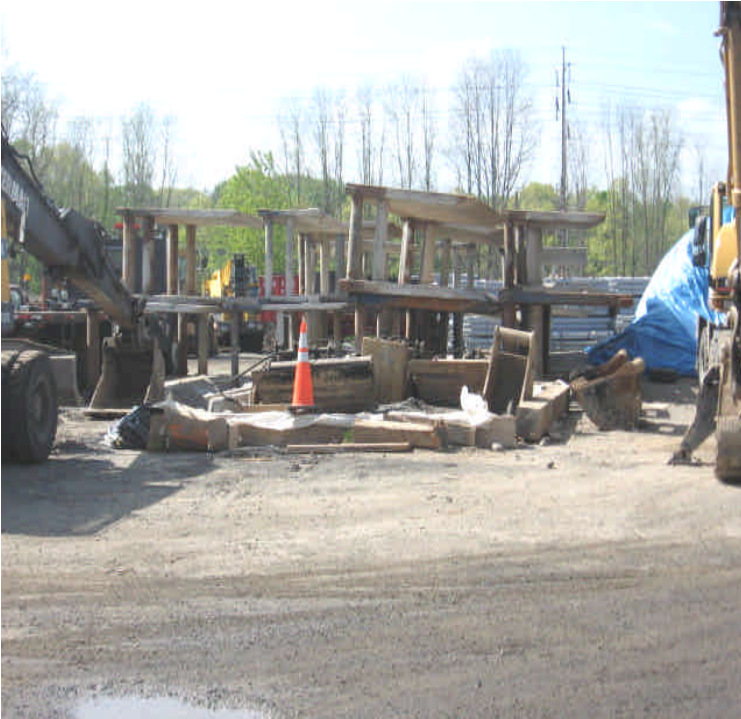
Fluid filled equipment is being adequately and proactively stored in a lined containment area.
