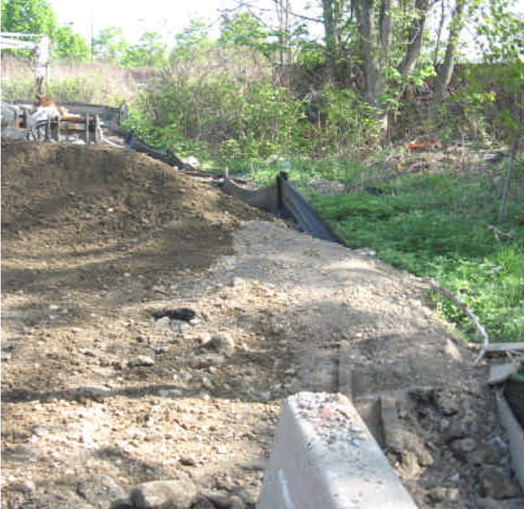
Material is overwhelming the perimeter controls in one location. Pull the soil back and restore the controls.
