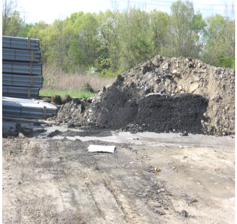
Slurry or concrete washout was deposited in an uncontained location within the yard. Concrete washout should occur in a proper containment area.
