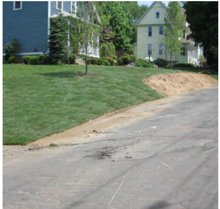
Turf has been applied to the majority of exposed soil and a tree was planted at the vault #3 location, in a good effort to restore the pre-construction conditions. Hay mulch remains on the remaining portion.
