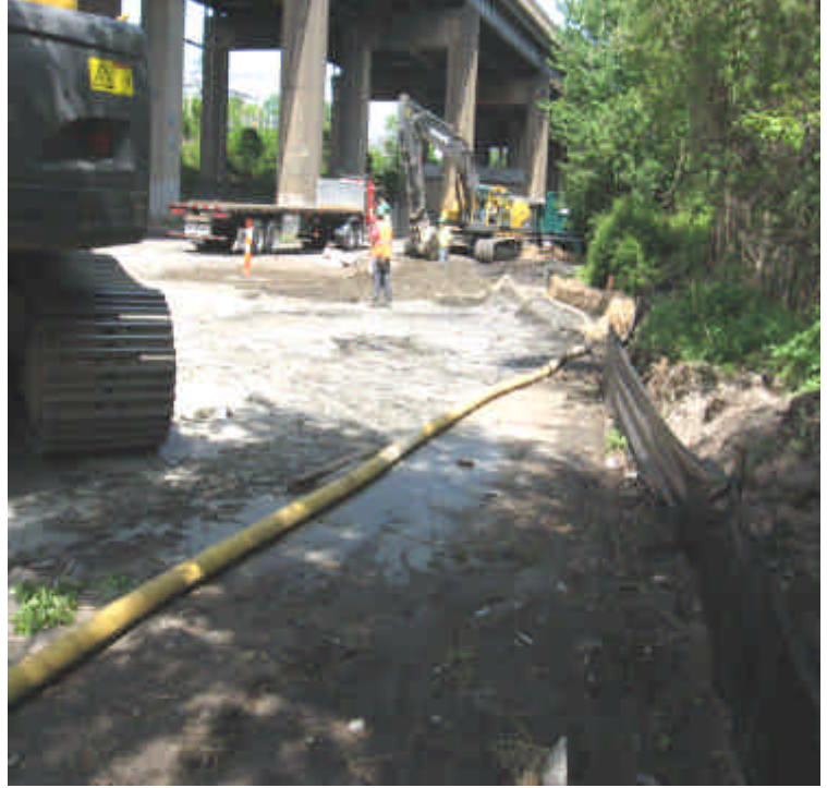
A film of flowable fill was observed on the pavement down-gradient of the vault location. This appears to be a result of groundwater interception with the construction activities.
