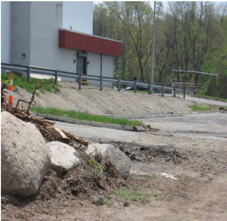
Photo of the exposed slope covered with hard-pack located near sta. #1076. Determine if the slope should be loamed and seeded to restore original conditions.
