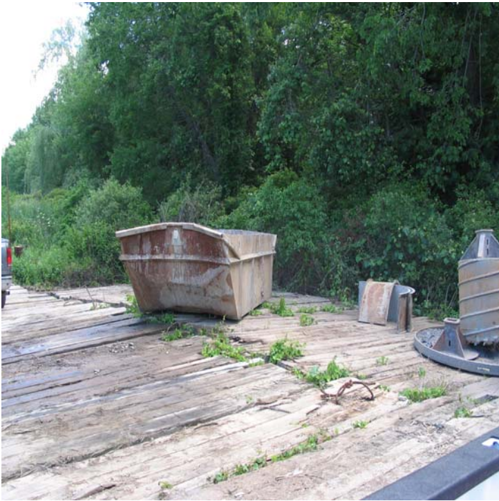
Ansonia Rd North (Woodbridge): Concrete is being washed to containment bins in this section.
