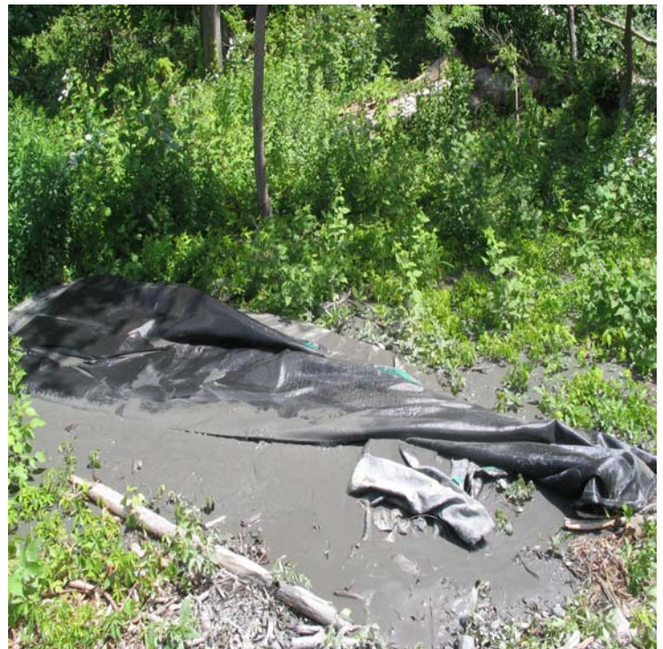
Pease Rd: Close up view of the filter bag at the dewatering area shown in the photo on the left. Sediment has escaped the controls here. The filter bag should be placed in a basin or surrounded by haybales to slow flow and increase filtration.
