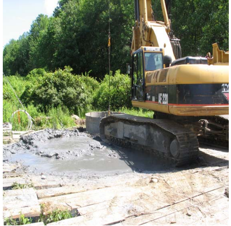
Manville Rd North (Woodbridge): Slurry was pumped directly to the timber mat crane pad here. Dewatering controls should be used at all times.
