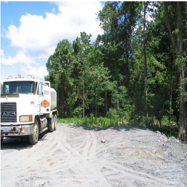
Pease Rd (Woodbridge): A view of the upland dewatering area here. Water is pumped from the truck to a filter bag at this location.
