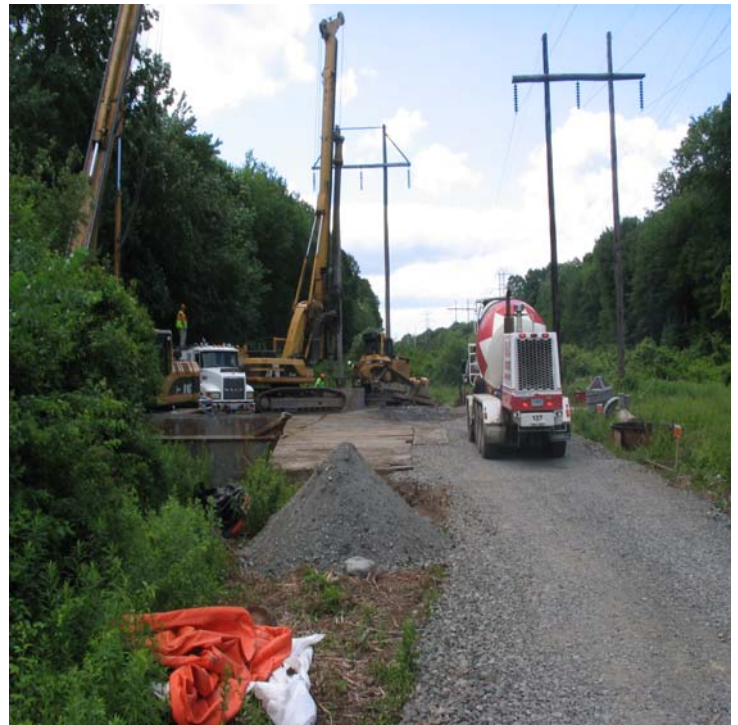
Ansonia Rd South (Woodbridge): Foundation drilling continues in this section. Water trucks were used for dewatering.
