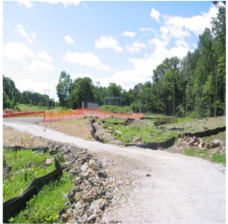
JCC (Woodbridge): Significant grass growth was noted in previously disturbed areas here. Erosion controls remain intact.
