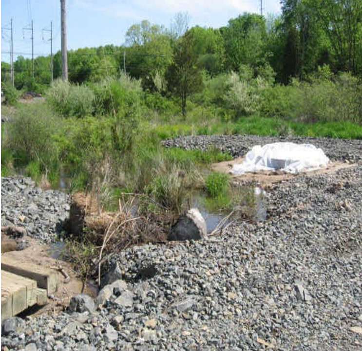
The foundation is in place within the wetland edge off Carpenter Lane. Place a filter sock between the exposed soil and the undisturbed portion of the wetland.
