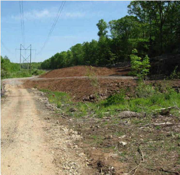
New pad site installed upgradient from a wetland crossing off High Hill Rd. Controls should be installed to contain exposed soil where needed.
