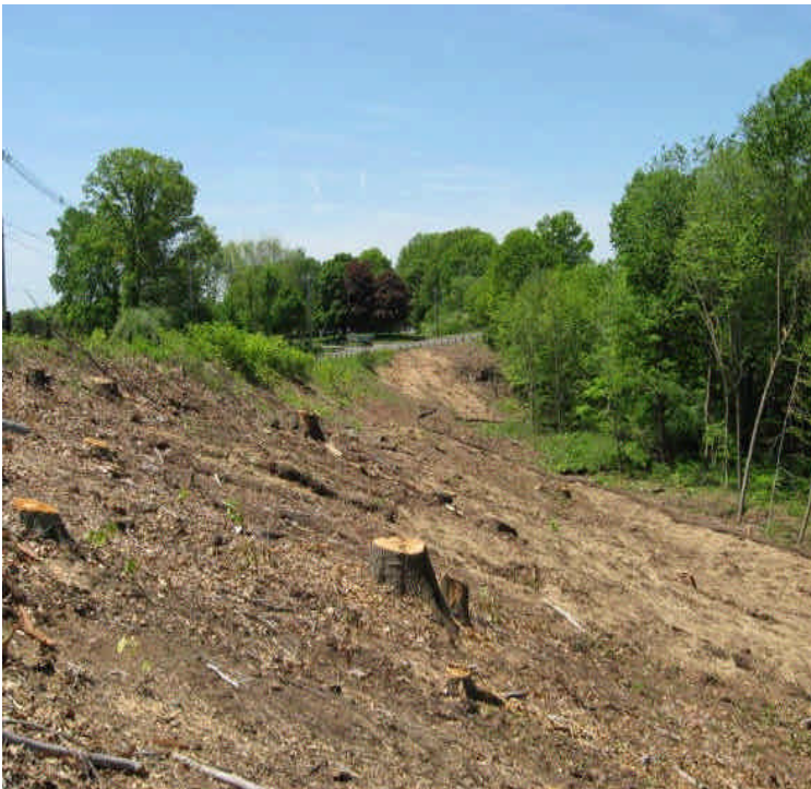
View of clearing off Harrison Rd. along a steep slope upgradient from a wetland. Hay and seed were placed along the slope
