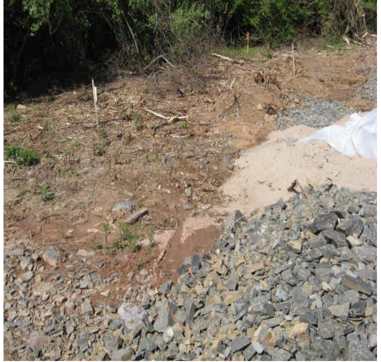
Slurry and sediment from a foundation had reached the edge of the and accumulated here against the haybales. Sediment over 2" deep should be carefully removed from the wetland by hand.
