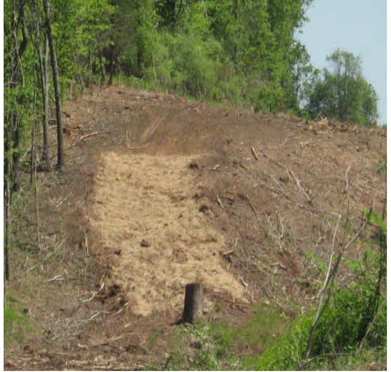
Looking toward Woodhouse Ave., new mulch placed on a steep slope upgradient from wetlands and Eastern box turtle habitat.
