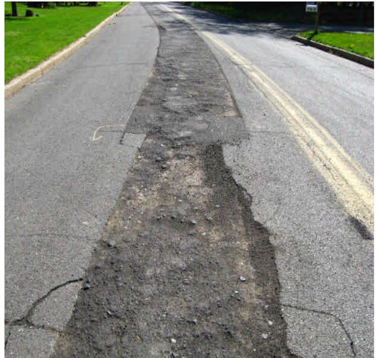
The asphalt patch along the trench along Old Farms Road is deteriorating and asphalt continues to crumble and accumulate along the roadway. Crews should finalize this surface as soon as feasible.
