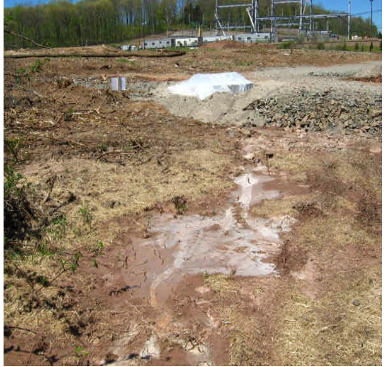
Slurry and sediment from a foundation had reached the edge of the and accumulated here against the haybales. Sediment over 2" deep should be carefully removed from the wetland by hand.
