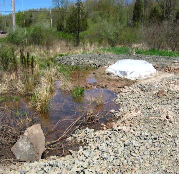
New foundation was installed within the wetland edge off Carpenter Lane. Place a filter sock between the exposed soil and the undisturbed portion of the wetland.
