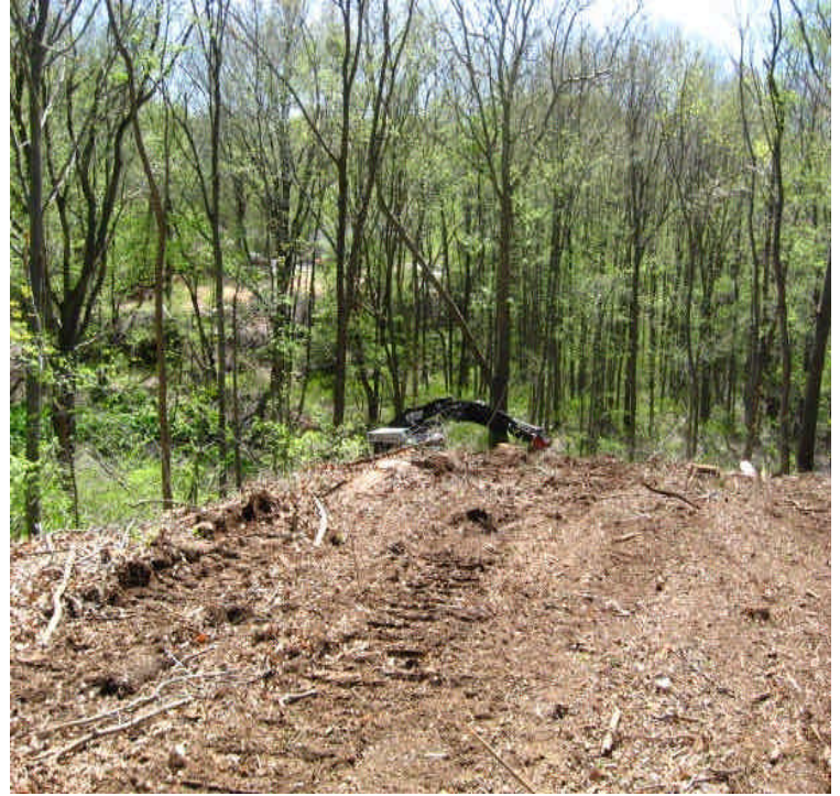
Clearing new ROW off Woodhouse Avenue on a steep slope adjacent to wetlands and previously unidentified Eastern box turtle habitat. Crews should now treat the area as habitat and perform turtle sweeps prior to equipment movement.
