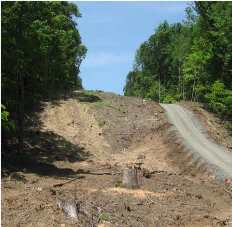
New access road installed, extending from the 1A connection off Black Walnut Drive.
