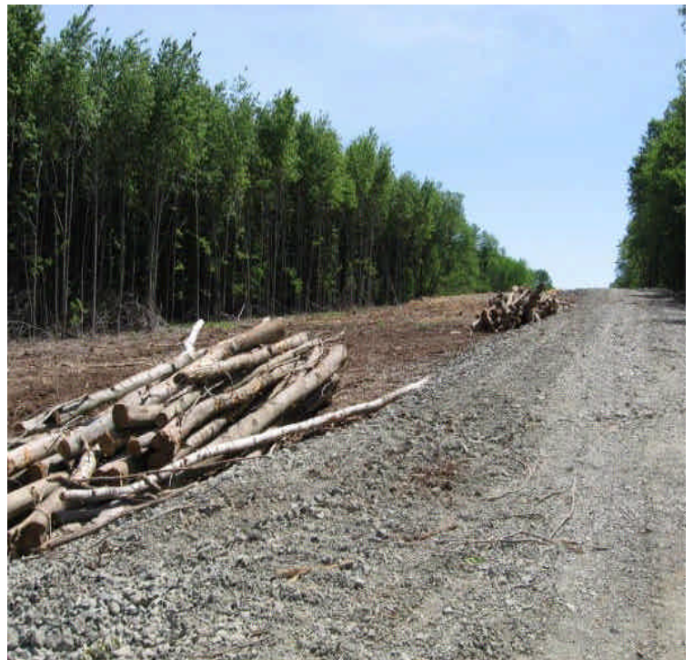
Tree stockpiles along the access, east of Rte 17. Attempt to retain native shrubs and vegetation wherever feasible.
