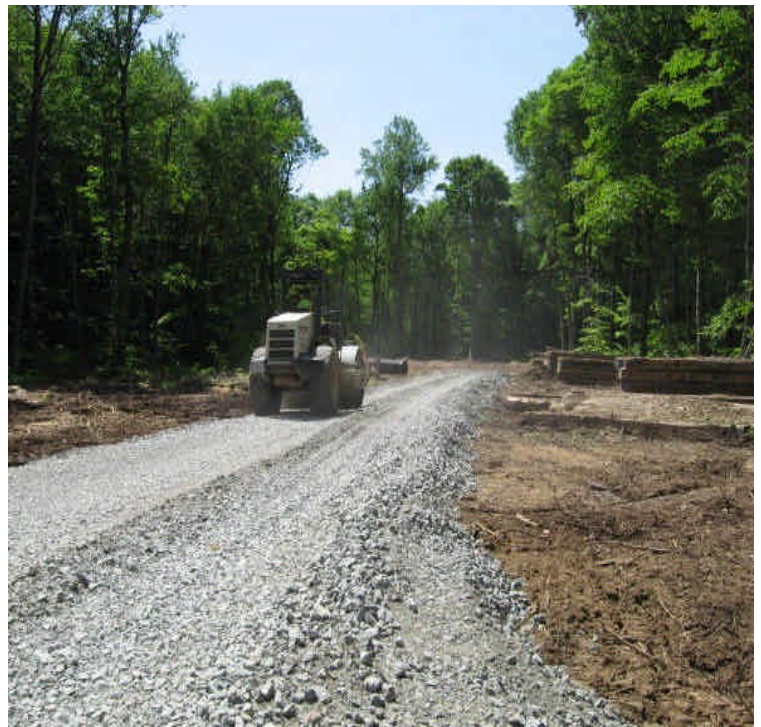
New access road construction into watershed protection area. Clearin has stopped at low impact area after the last pad site from this access.
