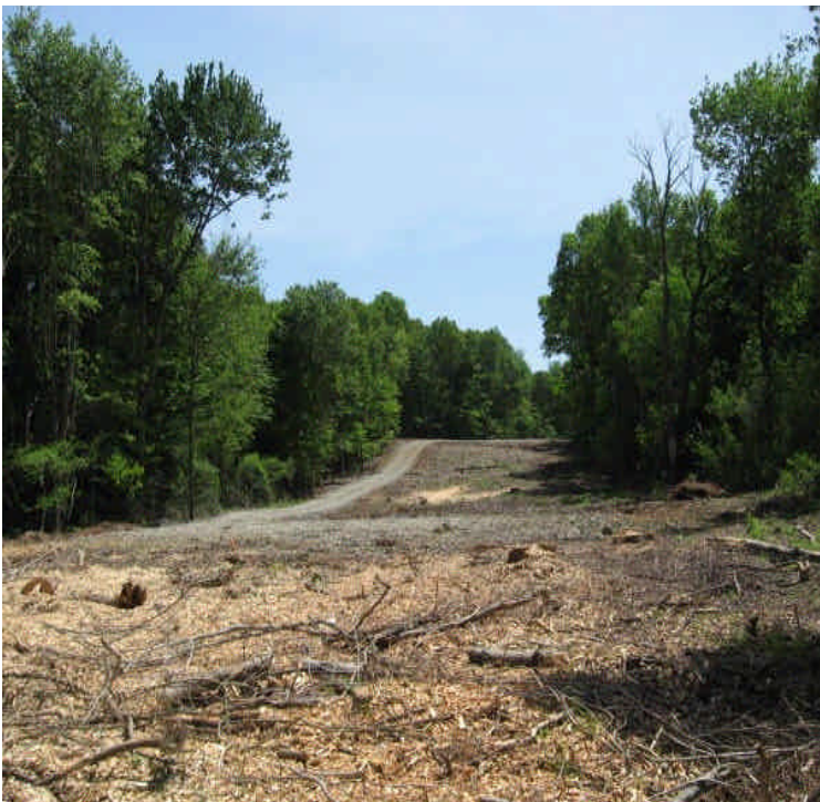
View of ROW clearing and pad construction looking toward the Segment 1A connection off Black Walnut Drive.
