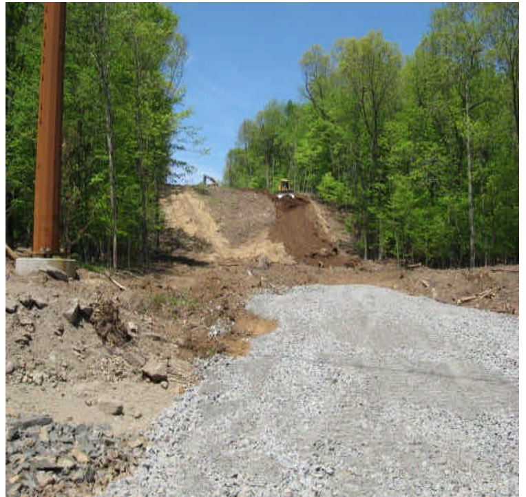
View of access road grading along a steep slope and installation of stone base. Controls such as erosion control blankets may be needed for stability/restoration here.
