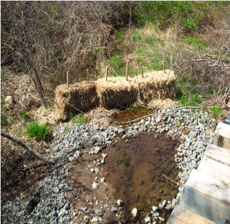
Stormwater controls remain adjacent to the timber mat crossing off Rte 17. Clear water was flowing off site.
