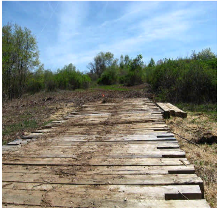
Hay mulch was spread at exposed soil along wetlands near Rte 17 to increase stability.
