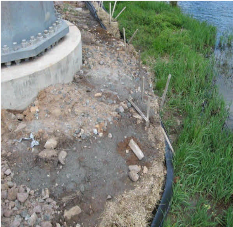
Controls remain in place along the pond north of Beseck SS to E. Meriden SS off Fleming Rd where pole installation is complete. However, sediment has filled controls to capacity immediately adjacent to the pond and needs to be removed
