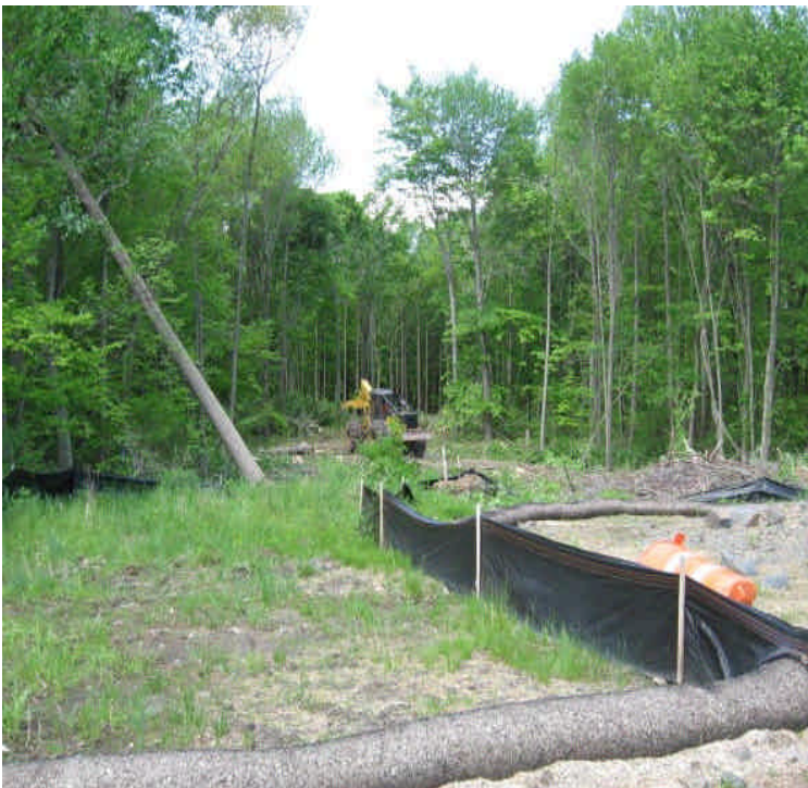
View of the controls and clearing at 1B from the contractor receiving yard.
