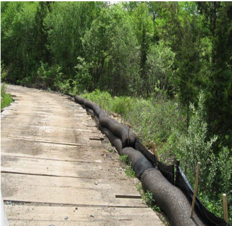
View of well installed haybales and fiber rolls at the timber mat crossing off Powder Hill Rd. Sediment is filtered from the run-off before it flows off-site in this area. Turbid water previously retained here has fully receded.
