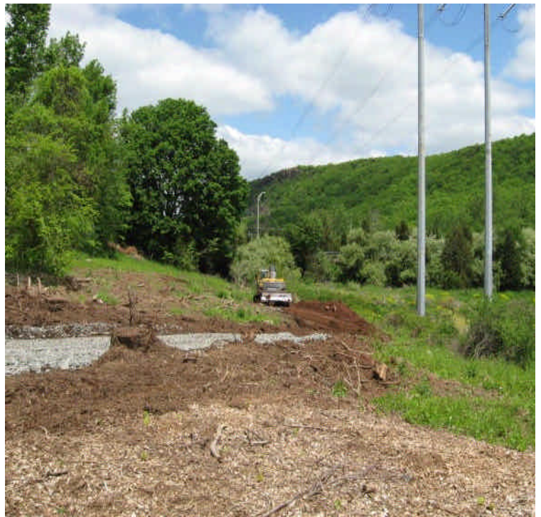
Site work north of East Main Street. Controls need to be extended as work continues.
