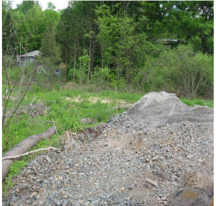
Sediment pile located on access road in wetlands south of High Hill Rd. Remove pile and locate all stockpiles away from wetlands.
