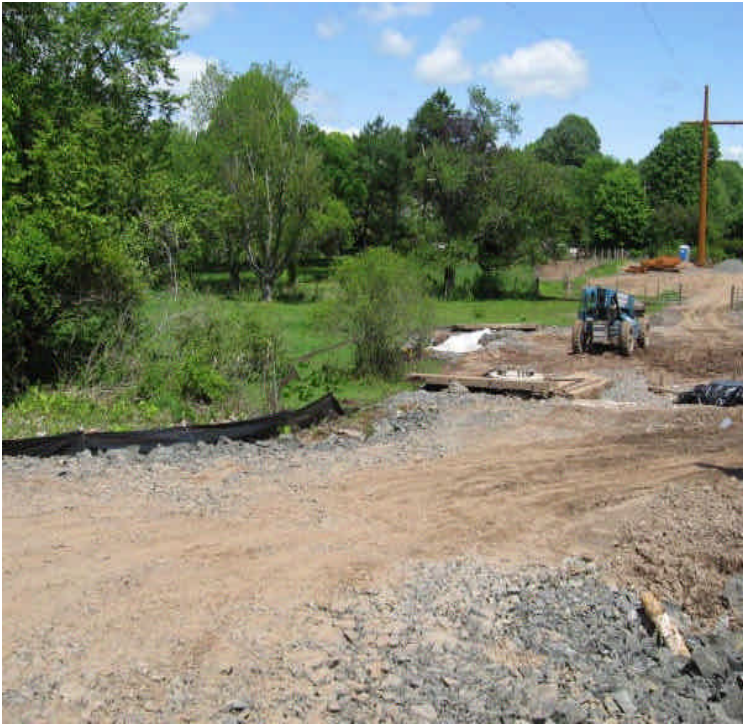
View of the controls at the wetland crossing off Little Lane.
