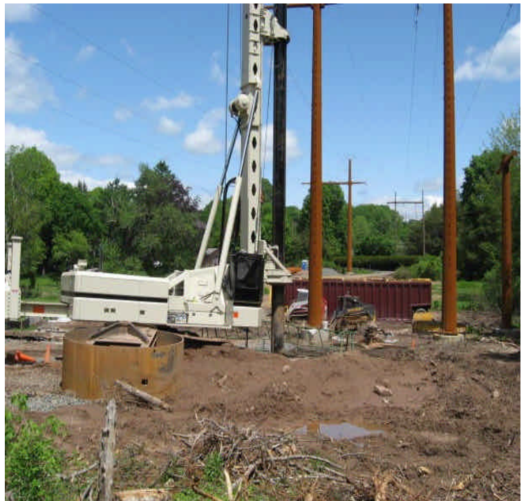
Permitted drilling was occurring within wetlands off Little Lane. A settling tank was in place for any slurry containment.
