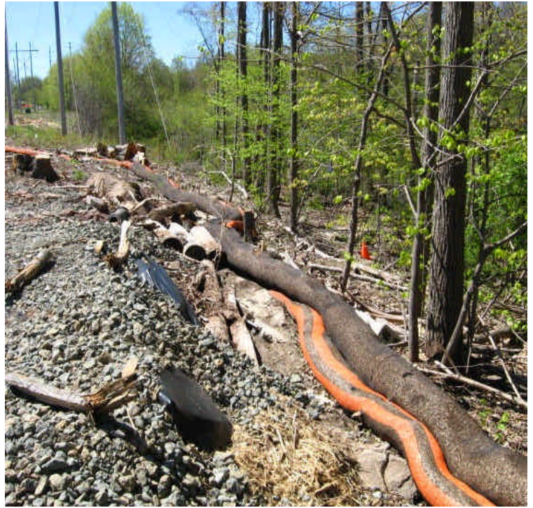
Filter socks just north of E. Meriden SS controls need to be toed in in order to work effectively. Haybales are in place at erosion prone areas for additional control.
