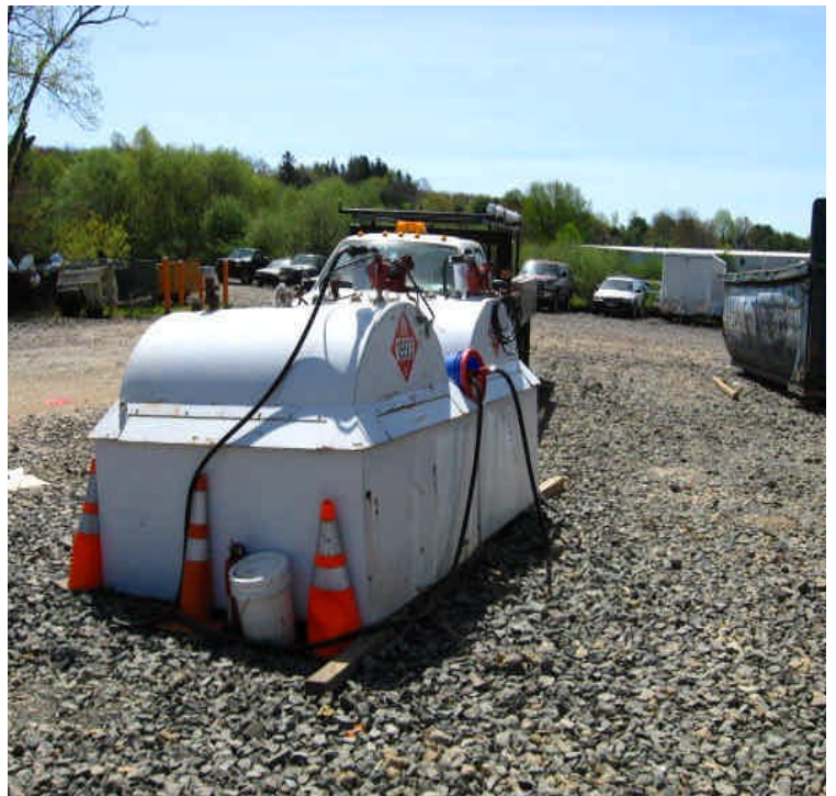
Both nozzles were well contained in a 5-gallon bucket within the contractor receiving yard.
