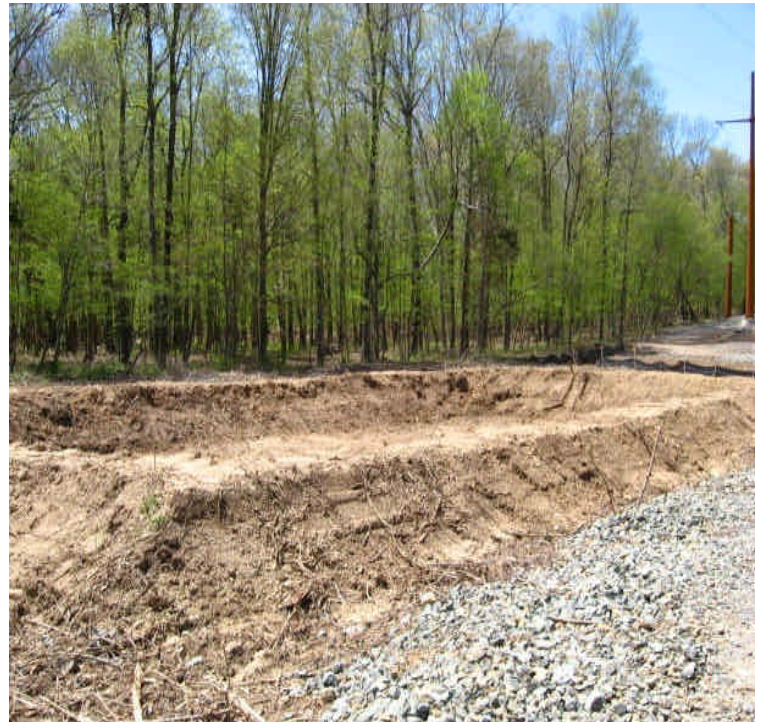
View of the basin in place off Black Walnut Drive upgradient from Ball Brook.
