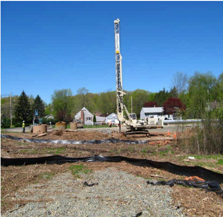
Foundation drilling upgradient from the wetlands just north of High Hill Rd. No sedimentation issues were noted; controls were in place.
