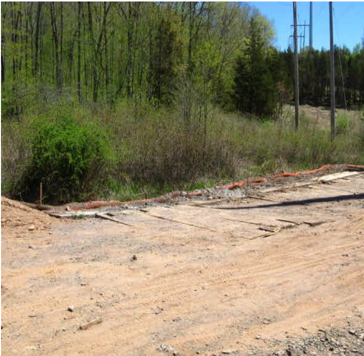
Sediment (likely from snow clearing) was noted on and beyond the filter sock at the matted pad near Beseck SS. Sediment in the wetland needs to be carefully removed by hand.
