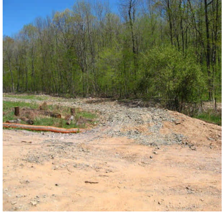
A line-pulling area north of Beseck SS has been graded and stone is in place to stabilize the area and reduce run-off. Haybales and filter sock barriers are in place for additional control.
