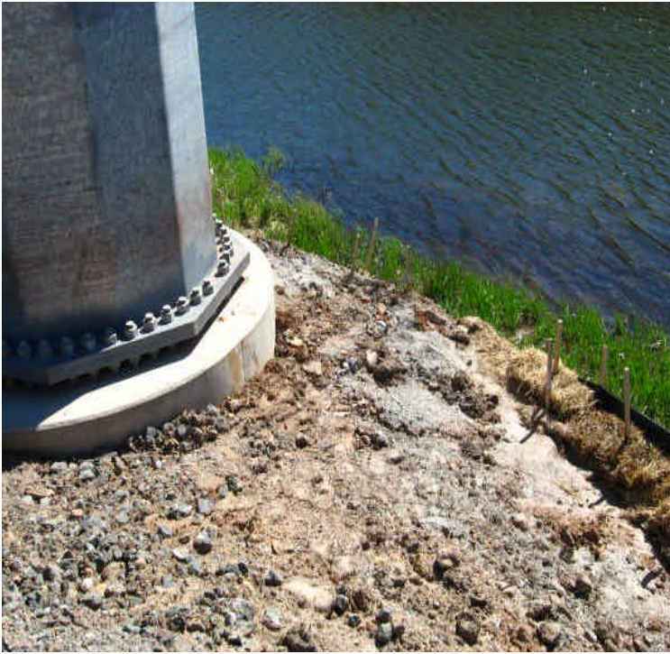
Controls remain in place along the pond north of Beseck SS to E. Meriden SS off Fleming Rd where pole installation is complete. However, sediment has filled controls to capacity and needs to be removed.
