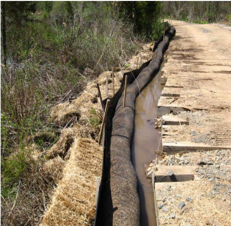
View of well installed haybales and fiber rolls at the timber mat crossing off Powder Hill Rd. Sediment is filtered from the run-off before it flows off-site in this area. A large amount of turbid water is still being retained here but is starting to recede.
