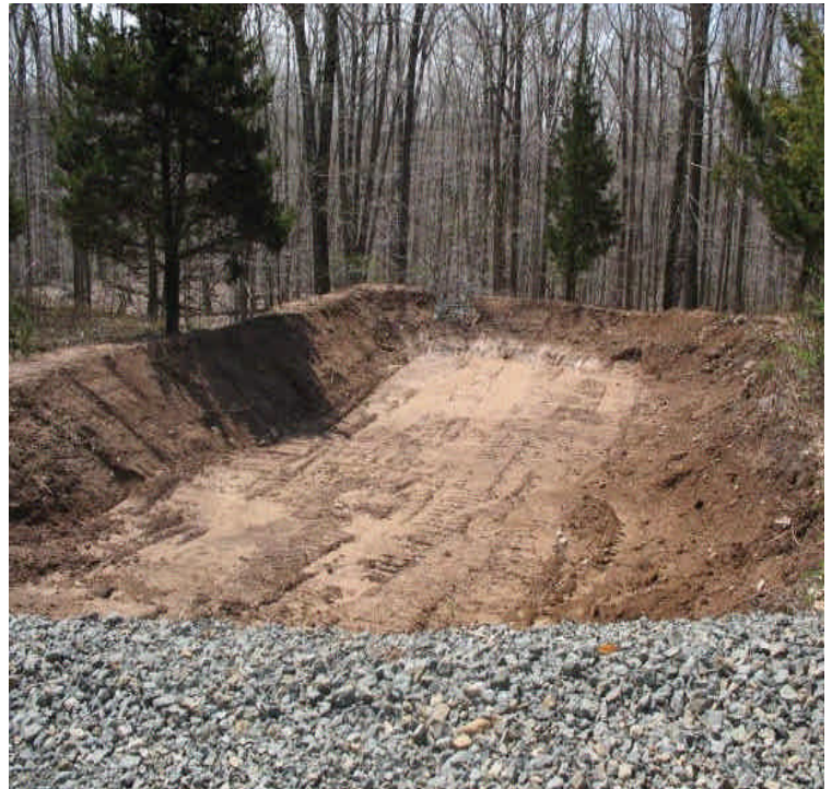
Detention basin in place off Black Walnut Drive upgradient of Ball Brook.
