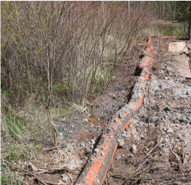
Sediment (likely from snow clearing) was noted on and beyond the filter sock at the matted pad near Beseck SS. Sediment in the wetland needs to be carefully removed by hand.
