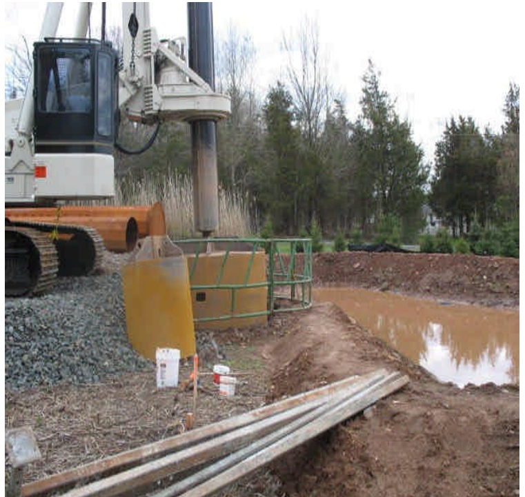
View of drilling east of Powder Hill Road. Detention basin in place to retain and settle run-off from the site.
