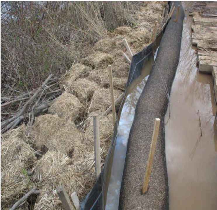
View of well installed haybales and fiber rolls at the timber mat crossing off Powder Hill Rd. Sediment is filtered from the run-off before it flows off-site in this area. A large amount of turbid water is being retained.
