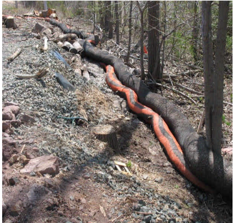
Filter socks just north of E. Meriden SS controls need to be toed in in order to work effectively. Haybales are in place at erosion prone areas for additional control.
