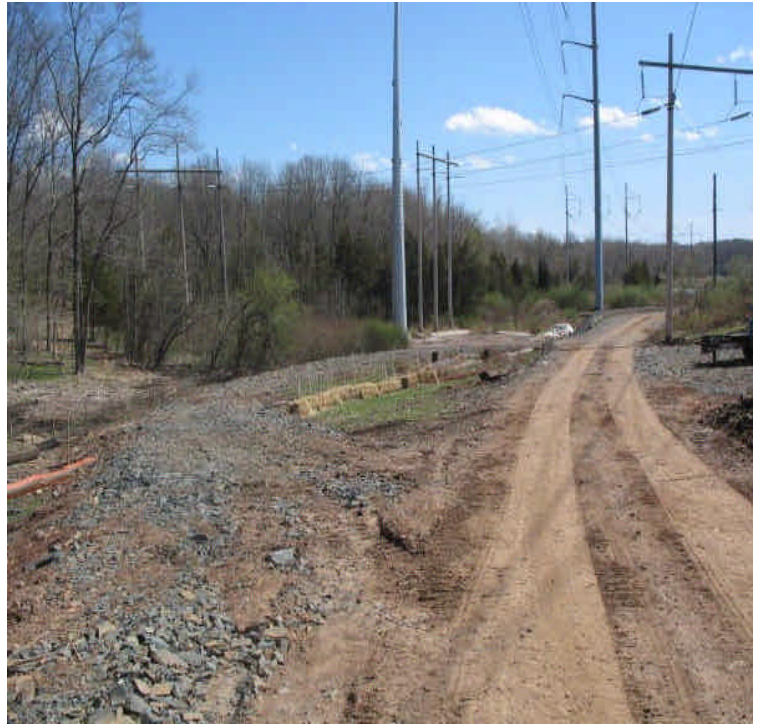
Access road north of Beseck SS is well controlled with stone in place to stabilize the soils and reduce run-off. Haybale and filter sock barriers are in place for additional control.
