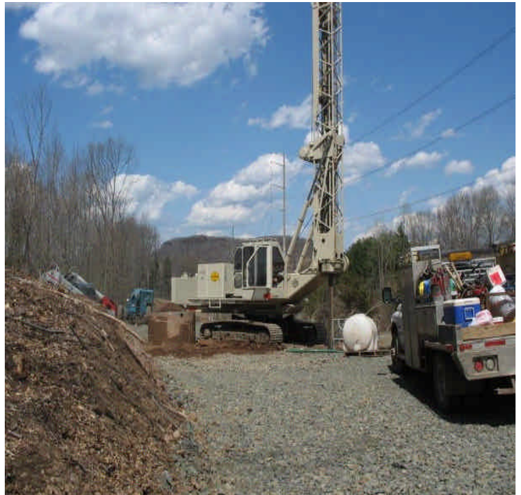
Foundation drilling north of High Hill Rd. near Black Pond. No sediment was noted entering the wetlands.
