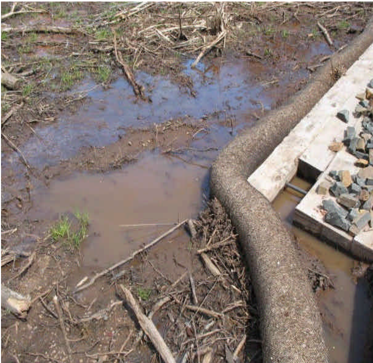
Foundation installed within the wetlands just south of High Hill Road. Slightly turbid run-off was noted leaving the timber mats under the filter socks but remained in the immediate area.
