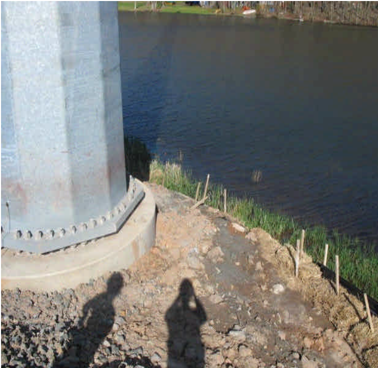
Controls remain in place along the pond north of Beseck SS to E. Meriden SS off Fleming Rd where pole installation is complete. However, sediment has filled controls to capacity and needs to be removed.
