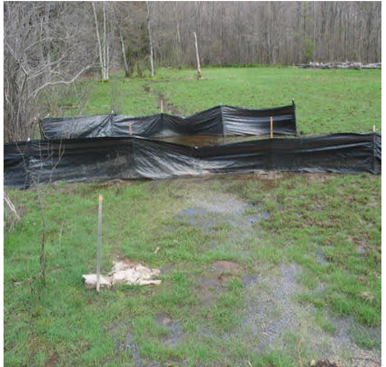
Area near the wetland crossing off Little Ln. Clear water was flowing through several lines of controls and off site.
