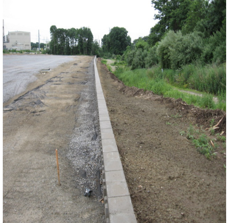
View of the completed retaining wall along the western boundary. Disturbed soils to the west of the retaining wall have been seeded. The mulch berm remains as a perimeter control here.
