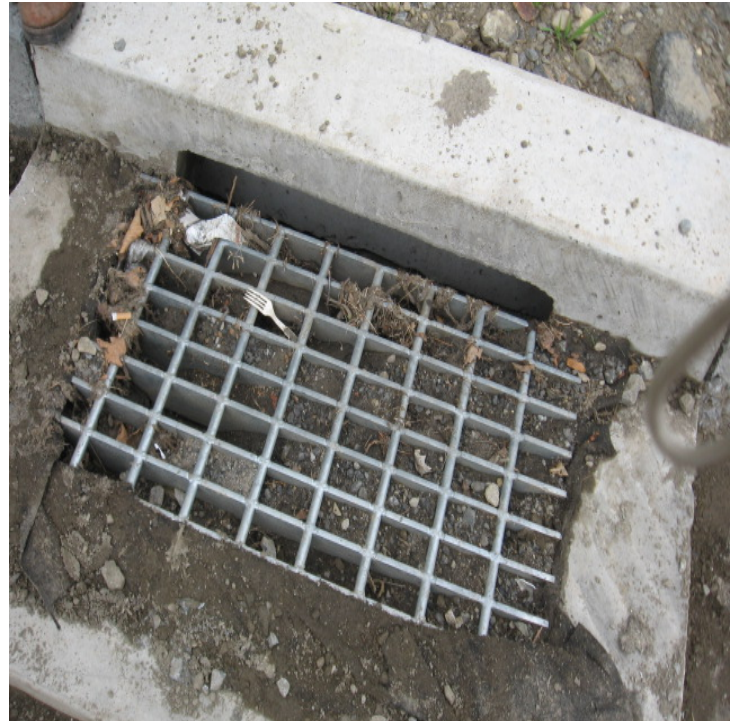
The "Silt sak" remains intact at the catch basin located at the corner of Shelland St. and Plains Rd, but curb inlet protection has not been provided.
