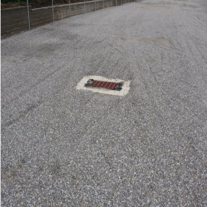
The catch basins along the western site boundary are now operational and "Silt saks" remain intact.
