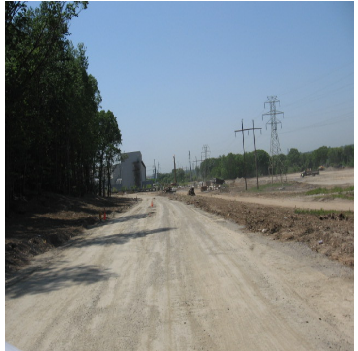
A view of the substation site from Shelland Street.
