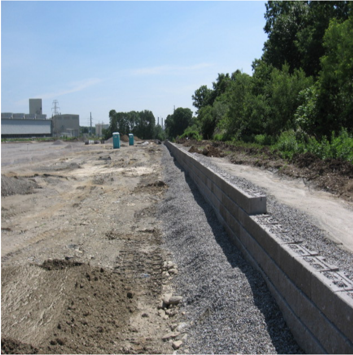
View of the perimeter/retaining wall along the western site boundary. Jersey barriers have been removed but wood chips remain.
