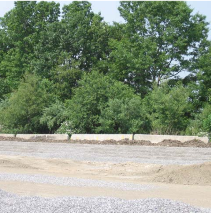
Retaining wall construction continues this week. Stone is still being spread throughout the site for dust control.
