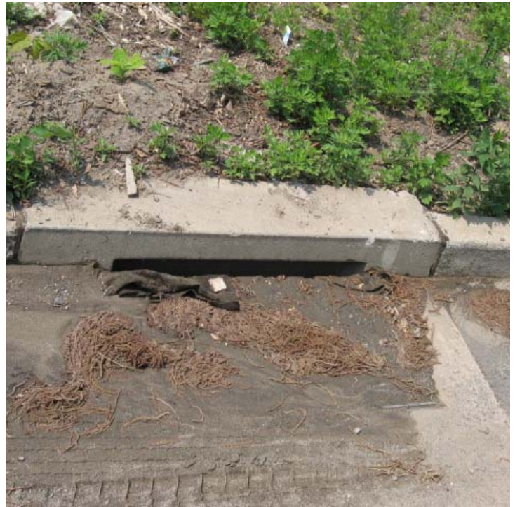
Sediment build up remains at some of the catch basins along Plains Road. Silt sacks remain intact but curb inlet protection was not provided in some locations.
