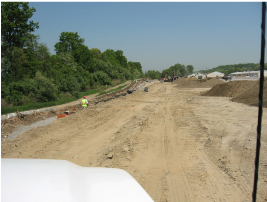
View of perimeter/retaining wall construction along the western site boundary. Stockpiles were noted here this week.
