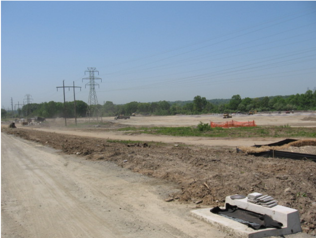
Overall view of substation work from Shelland Street. Site grading and stone spreading continues.
