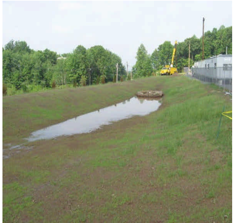
Haybales and controls remain in place at the inlet of the detention basin. Some run-off has ponded here. Additional grass growth was noted in recently hydroseeded areas.
