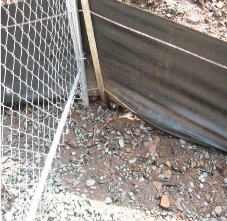
Silt fence at entrance off Carpenter Lane appears to have been undermined by stormwater run-off and should be toed back in.
