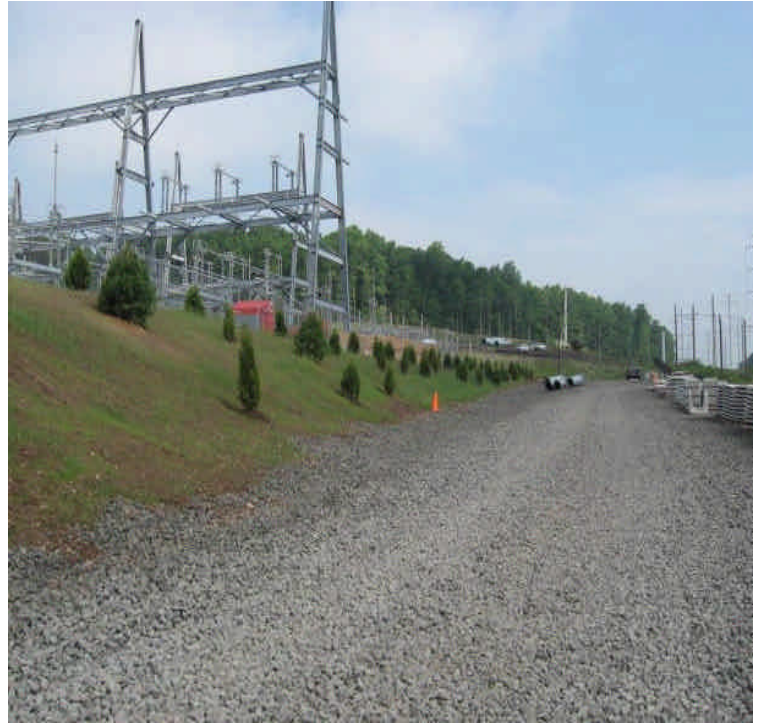
View of the eastern site exit and shrubs in place along the slope. Grass cover also appears to be increasing here.
