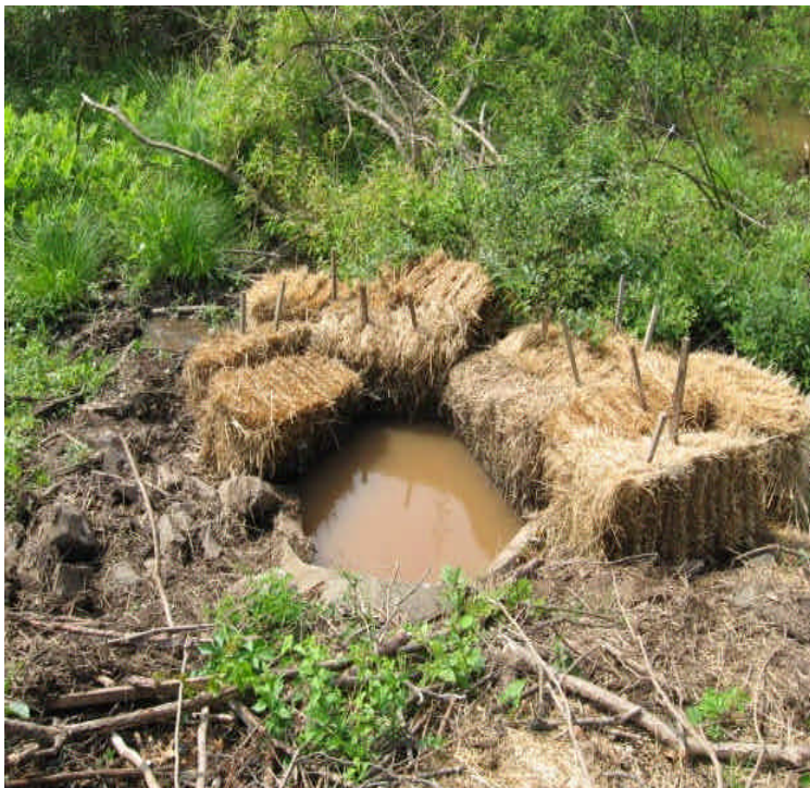
Storm drain outlet across Carpenter Lane has standing turbid water as a result of the storm and some site run-off
