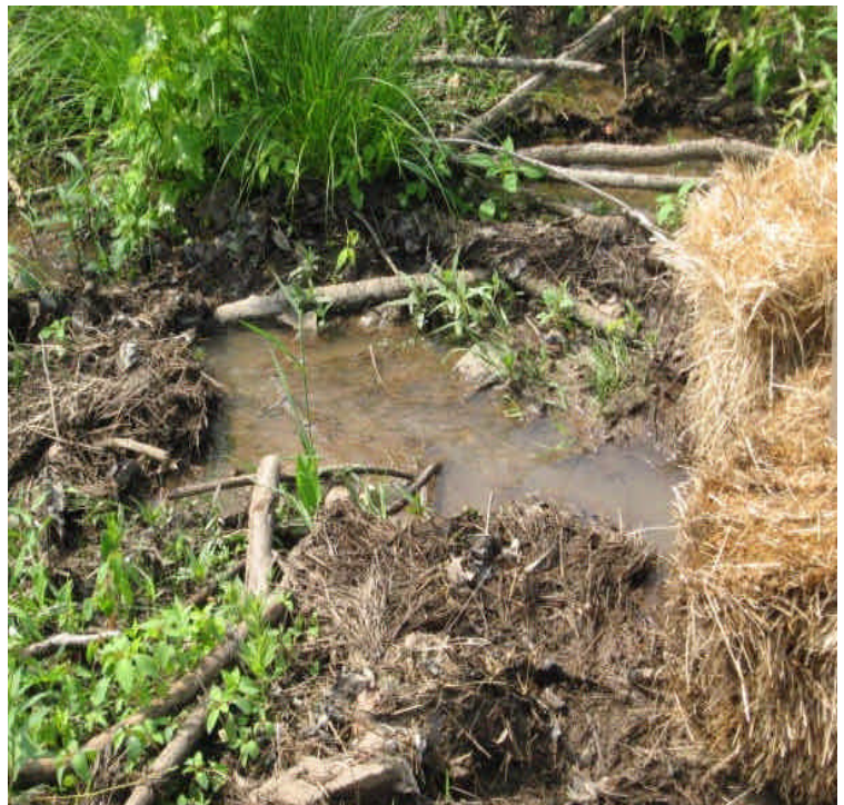
Mostly clear water was observed leaving the haybales and entering the wetlands. The new haybales helped to filter out the sediment. Evaluate whether the amount of sediment accumulation justifies the minor disturbance needed to remove it, once the water subsides.
