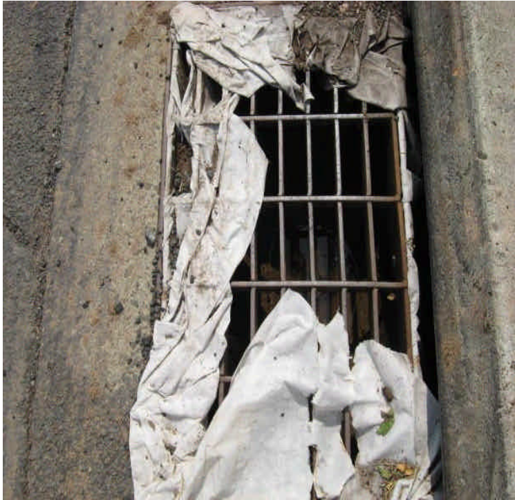
Clean and replace CB controls along Carpenter Lane. They had deteriorated as a result of the rain event.
