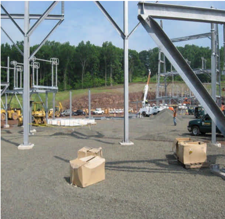
View of the entire site from the southeast corner looking north Stone is being spread at completed areas for further stabilization
