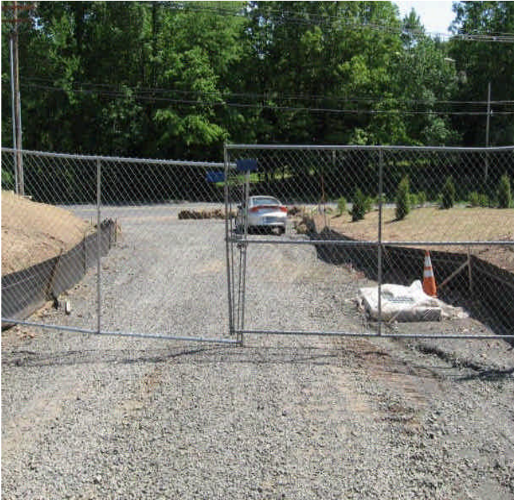
Site entrance off Carpenter Lane is at final grade. Stone base and stone check dams remain in place.
