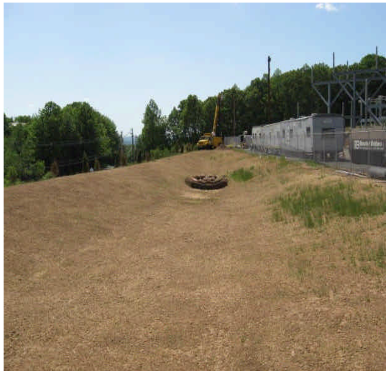
Haybales and controls remain in place at the inlet of the detention basin. Basin slopes and floors have been graded and hydroseeded.
