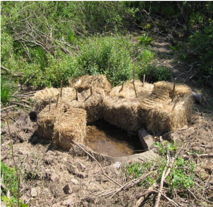
Storm drain outlet across Carpenter Lane has clear water flowing through the haybales. Deteriorated haybales were removed and replaced.
