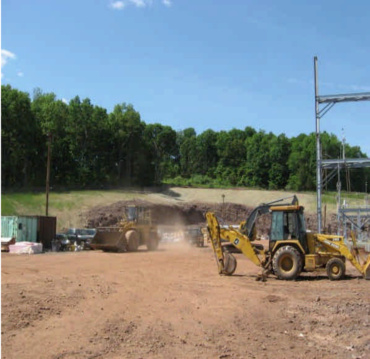
Some airborne dust generation was noted; Continue to monitor and add controls as needed
