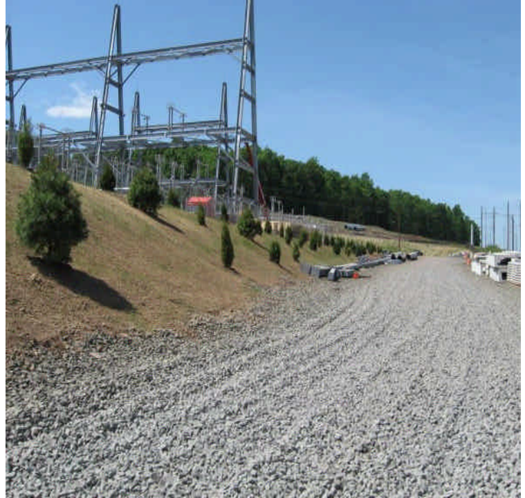
View of the eastern site exit and the new shrubs planted along the slope.
