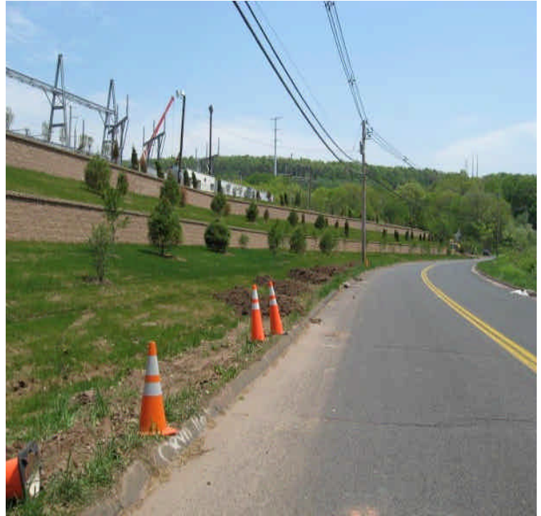
Silt fence was removed along Carpenter Lane. Apply seed to any exposed soil resulting from the removal.
