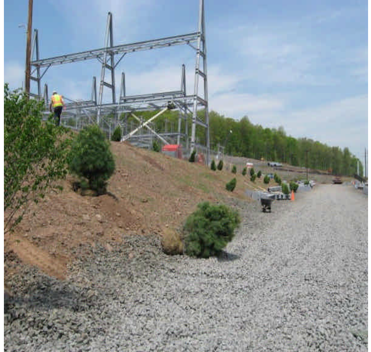
View of the eastern site exit and new shrubs being planted along the slope. Consider adding more seed along the slope as well.
