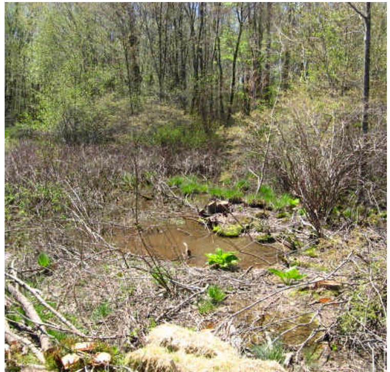
Clear water was observed leaving the haybales and ponding in the wetlands. Evaluate whether the amount of sediment accumulation justifies the minor disturbance needed to remove it, once the water subsides.
