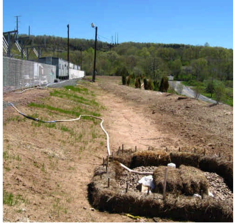
Haybales and controls remain in place at the inlet of the detention basin. Clean water from the frac tank was being discharged directly to the inlet.
