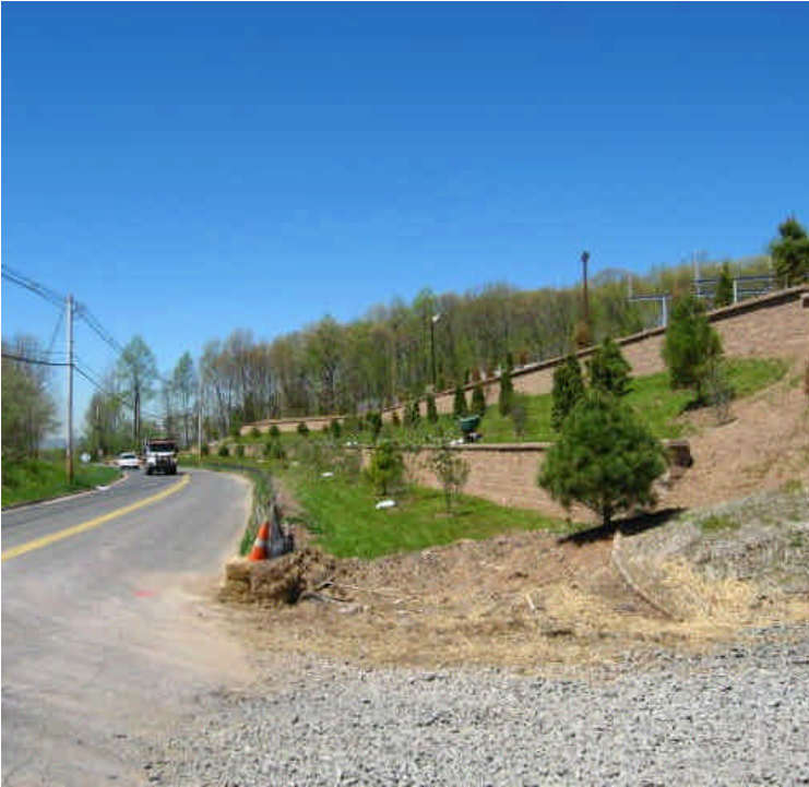
Site egress off Carpenter Lane had minimal sediment tracking but; no turbid run-off. Haybales should be replaced for run-off containment.
