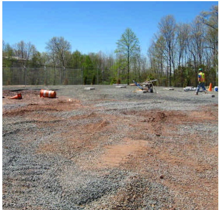
Stone was being spread in some of the areas where structure foundations were complete for additional stabilization on site.
