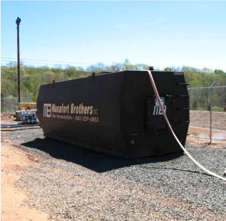
A frac tank was being used on site to hold and settle-out water from foundation excavations.
