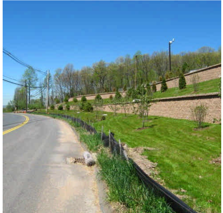
Some sediment accumulation remains in the gutter of Carpenter Lane. Continue to sweep by hand if necessary.
