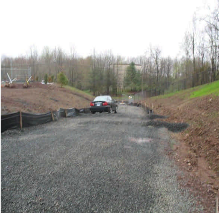
Stone base and stone check dams remain in place along the site entrance.
