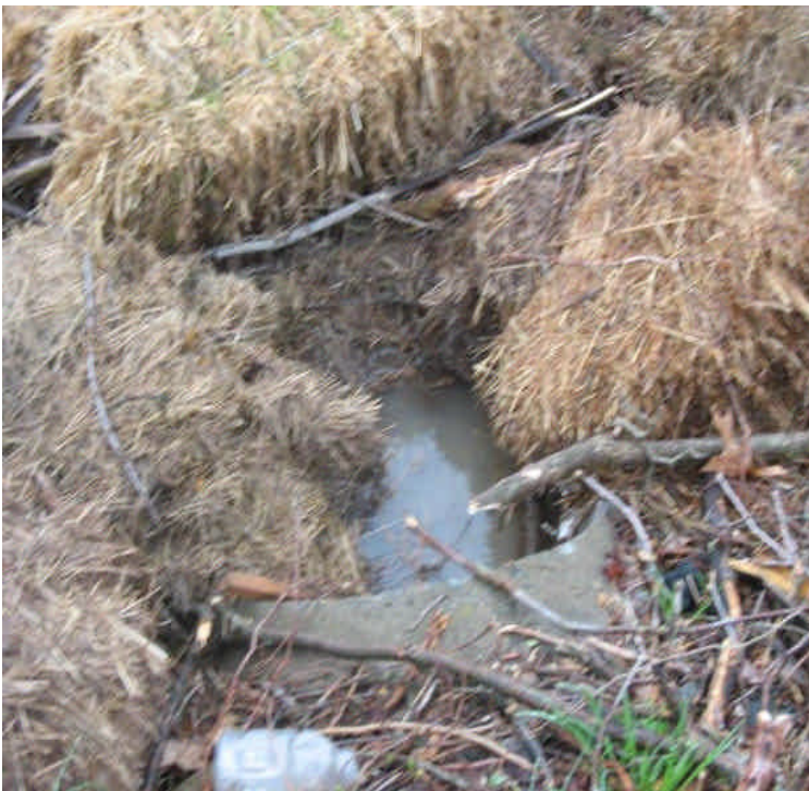
Storm drain outlet across Carpenter Lane has turbid water flowing through the haybales.
