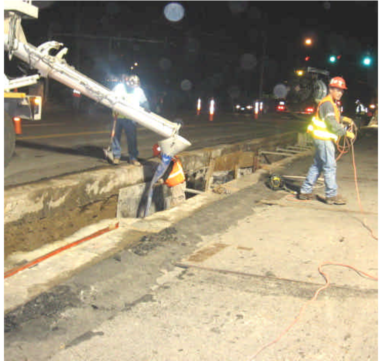
View of crews backfilling the trench located at sta. #195 to 197. A vac truck was dewatering the opposite end of the trench in the background of the photo.
