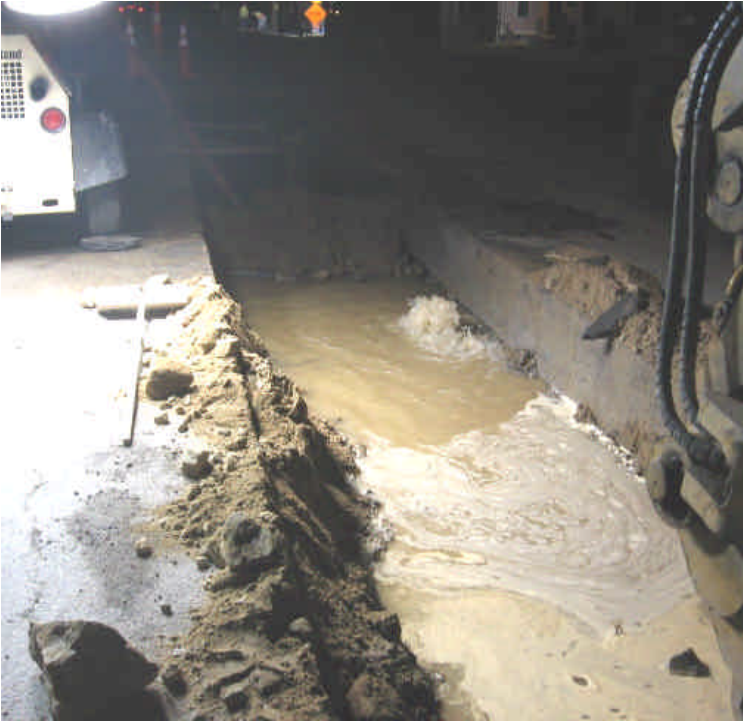
During trenching activities at sta. #226 to 228, the crew hit a water main that delayed construction. All water remained contained to the trench.
