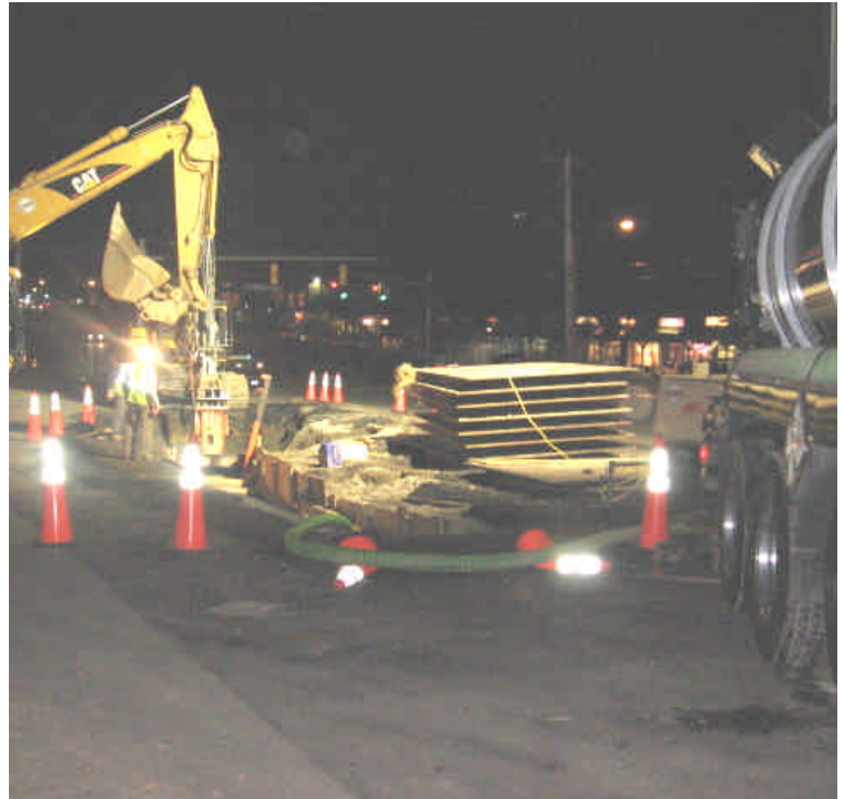
Trenching activities at vault #18 required dewatering. A vac truck was used appropriately.
