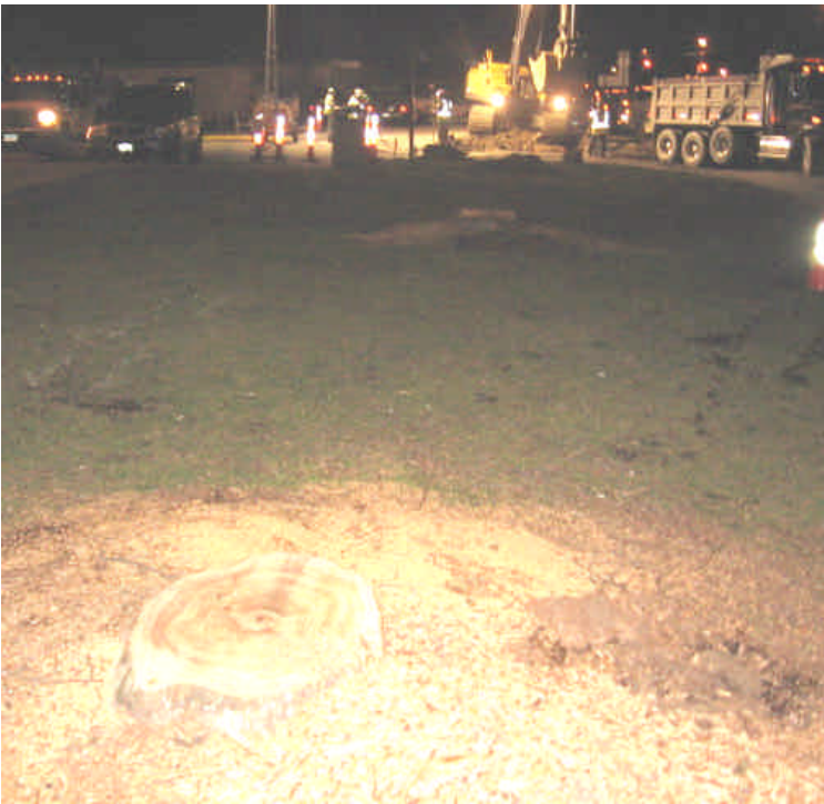
Five trees were removed south of vault #20 to accommodate trenching activities, and as approved by the D&M Plan.
