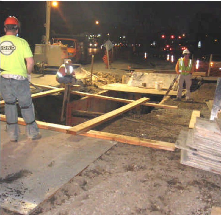
Trenching activities were being conducted at numerous locations along the project route.
