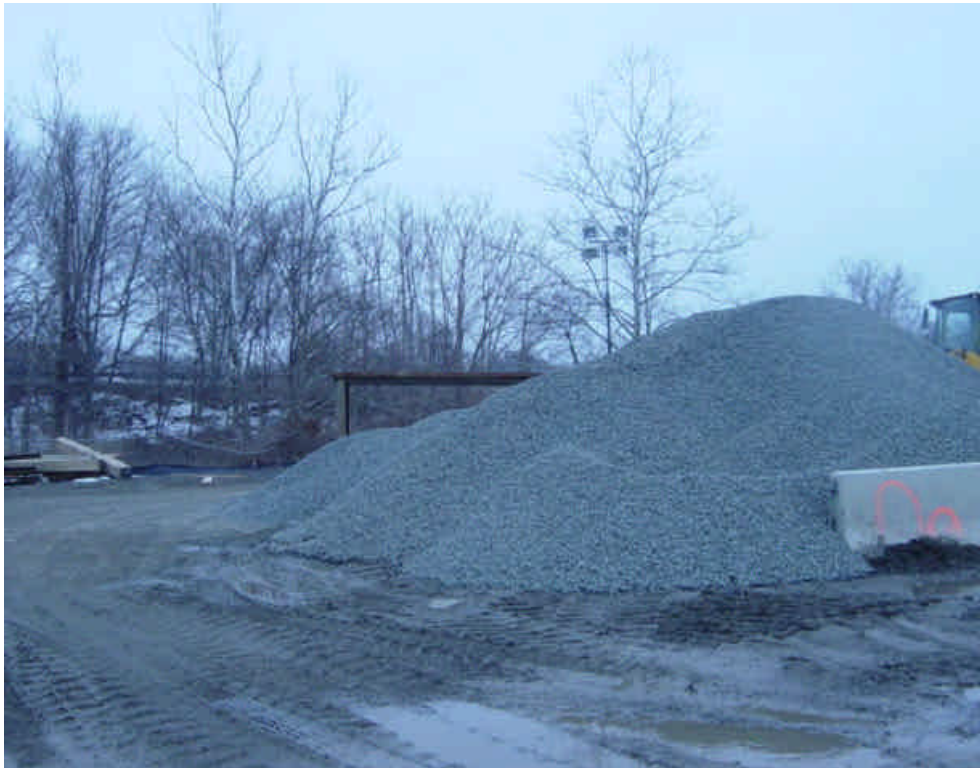
Concrete washout basin materials have been removed from the Kings Highway lay-down yard (off Kings Highway, near Rt. 1 rotary). Materials are contained within the yard.
