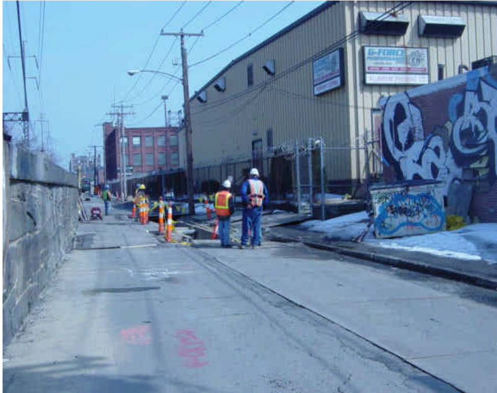
View of trenching activities within Railroad Ave. between Rt. 1 and Bostwick Ave.
