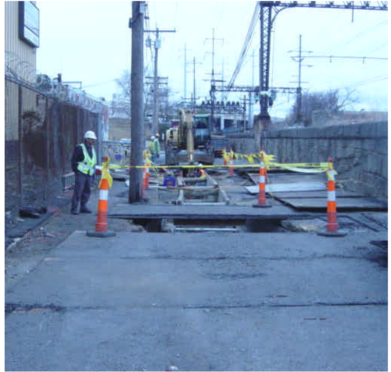
View of trenching activities within Railroad Ave. between Rt. 1 and Bostwick Ave.
