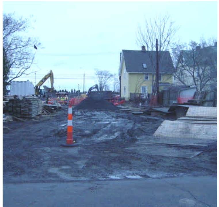
Trenching activities between Broad and Main St. No tracking was noted on either of the roadways as a result of the work.
