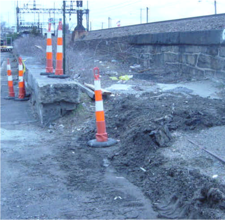
Concrete washout has been released in an uncontained location on Railroad Ave. between Rt. 1 and Bostwick Ave.
