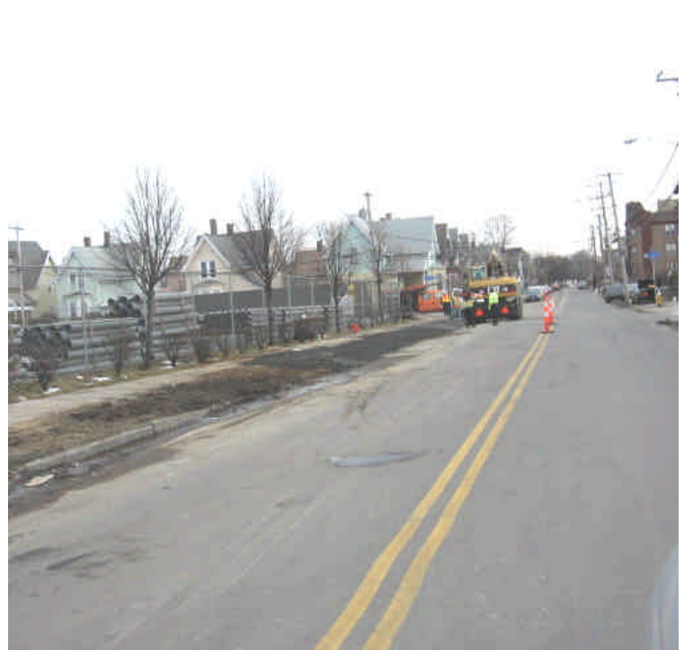
The roadway shoulder on Broad St. is being restored with aggregate as the trench is backfilled. The decision was made to use aggregate to prevent rutting along the roadway after this issue was noted along Railroad Ave.
