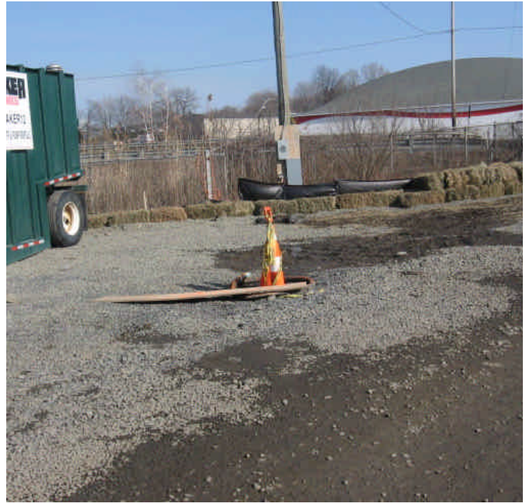
Perimeter erosion controls have been re-established proactively in the King Highway lay-down yard.
