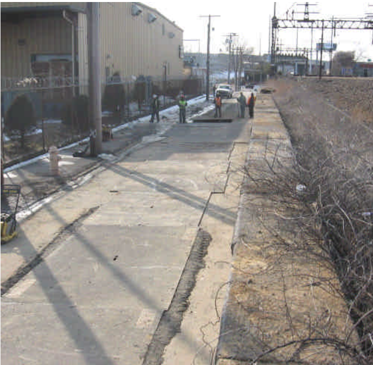
Trenching activities being conducted on Railroad Ave. between Rt. 1 and Bostwick Ave.
