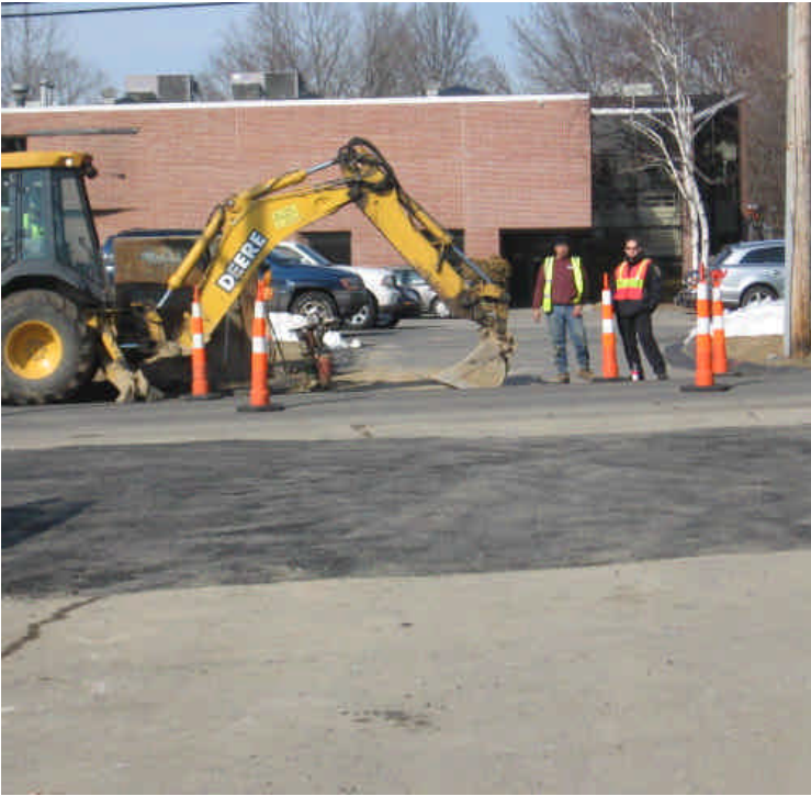
Utility work being conducted adjacent to Vault #28. Continue to sweep pavement as necessary.
