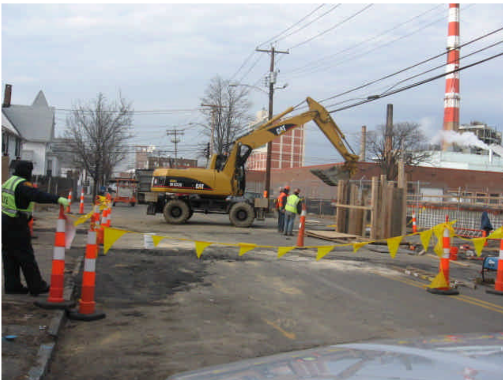
View of trenching activities on Main St. Sediment tracking was noted along the roadway; Street sweeping should be performed.
