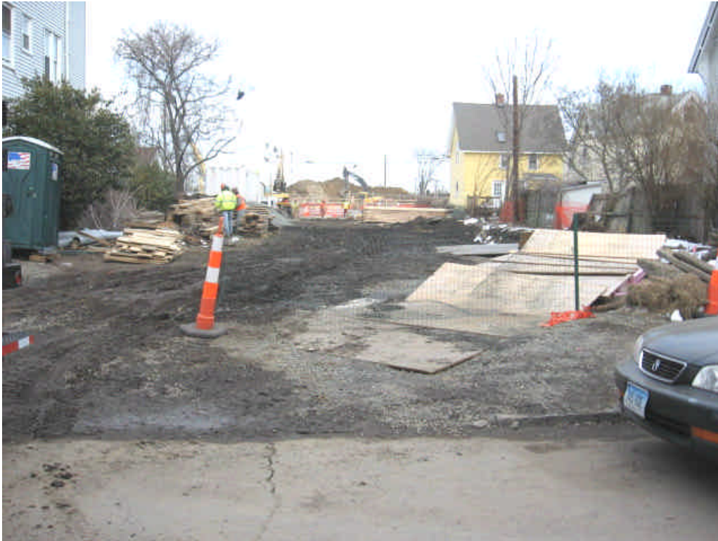
Trenching activities between Broad and Main Sts. Some sediment tracking was noted on Broad St.; Street sweeping should be performed.
